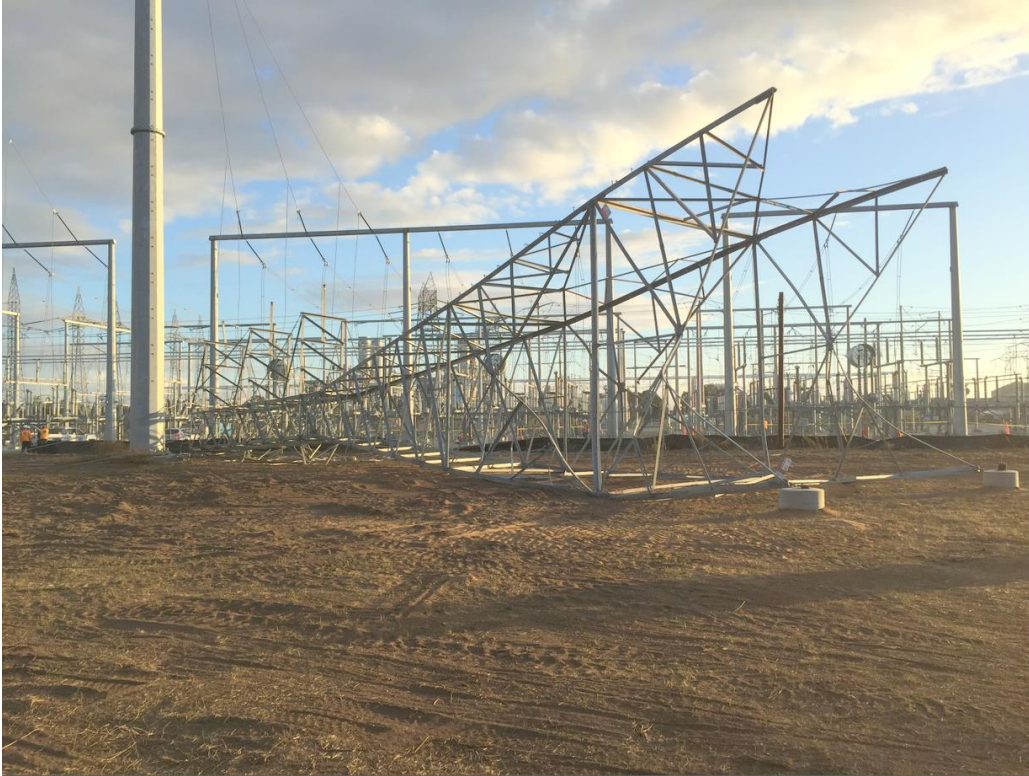
Figure 1: Moss Landing Tower Collapse Site Photo
