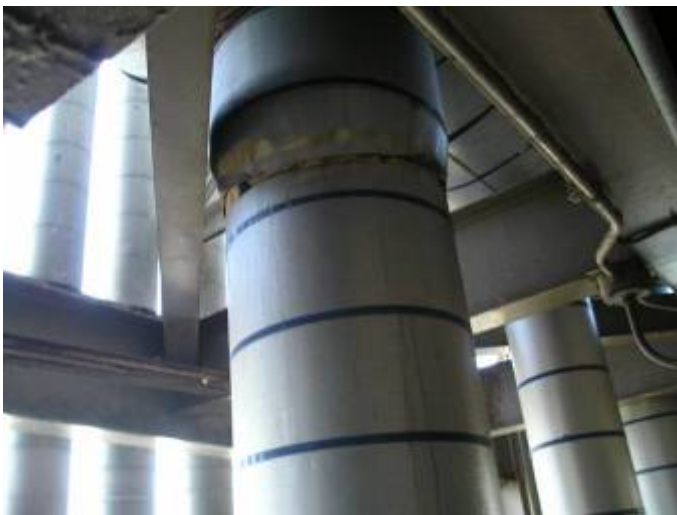
Figure 14. Pipe missing insulation.
