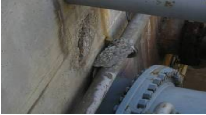
Figure 13. Fallen concrete rests on a pipe.
