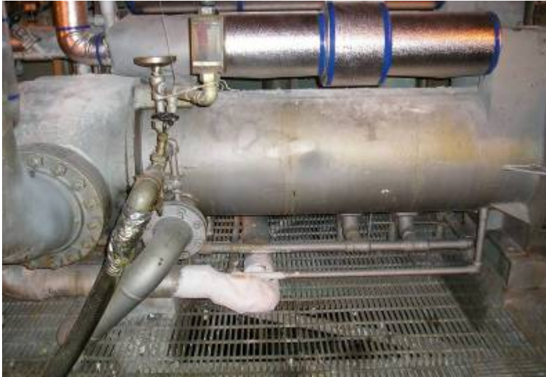
Figure 4. The plant taped a hose to the steam jet air ejector to exhaust fumes.
