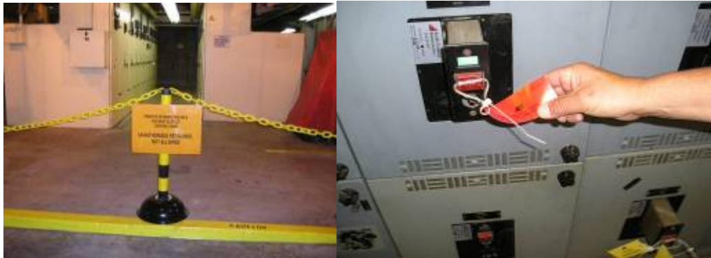
Figure 17. Auditors saw warning signs and equipment clearance tags throughout the plant.
