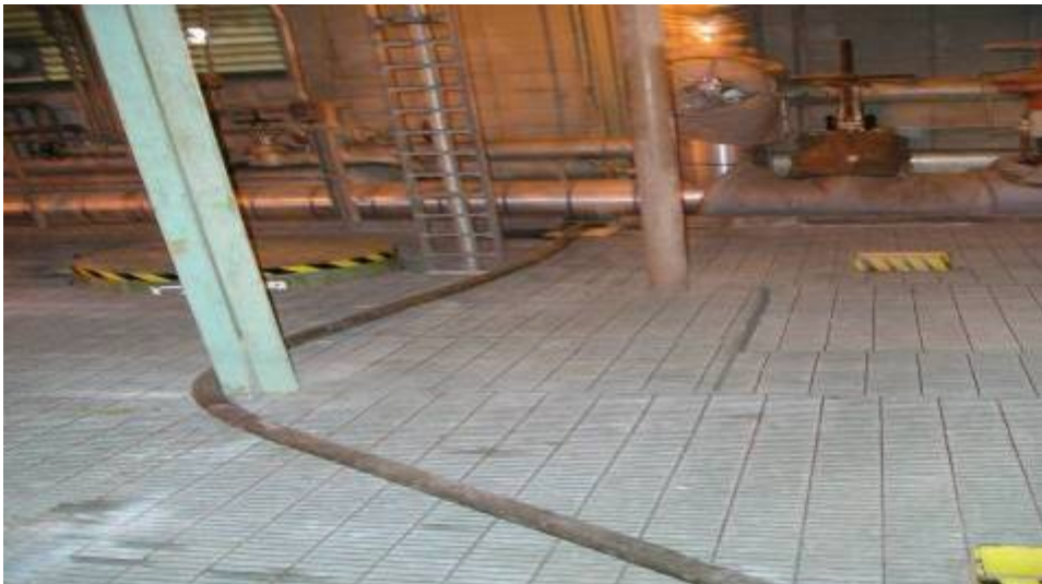
Figure 5. The hose from the steam jet air ejector extends through the auxiliary bay.
