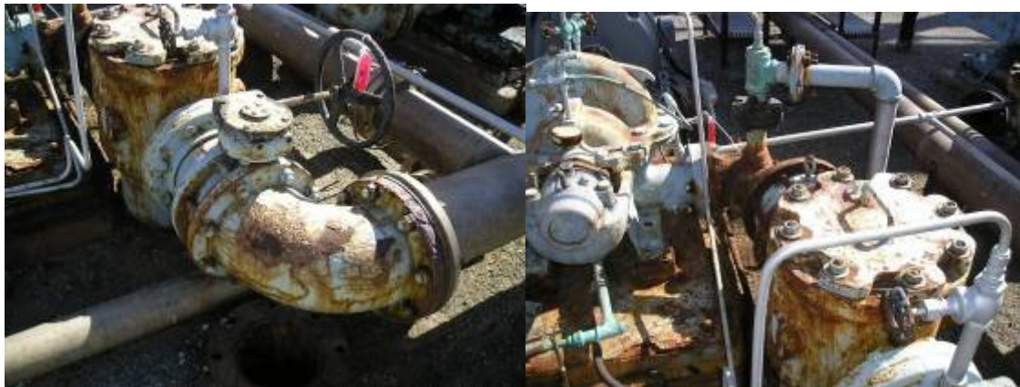
Figure 2. Corrosion at the plant.
