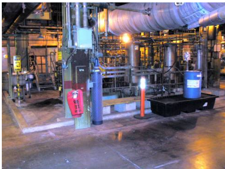
Figure 8. Hydrazine area after the metal tote and excess (blue) hydrazine drums were removed.
