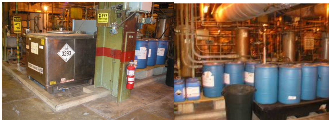
Figure 3. Hydrazine mixing and storage area appears capable of storing over 100 gallons of hydrazine.
