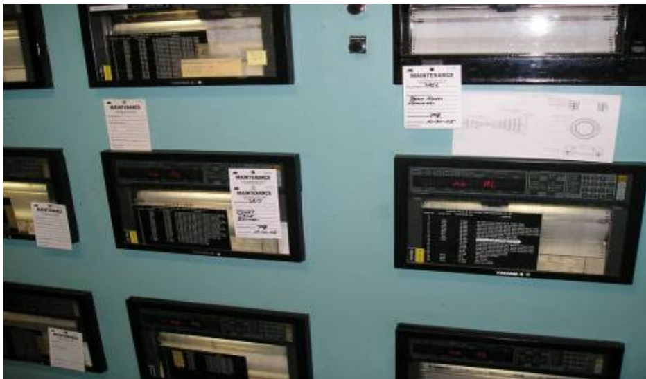
Figure 10. Chart recorders in control room need repairs.
