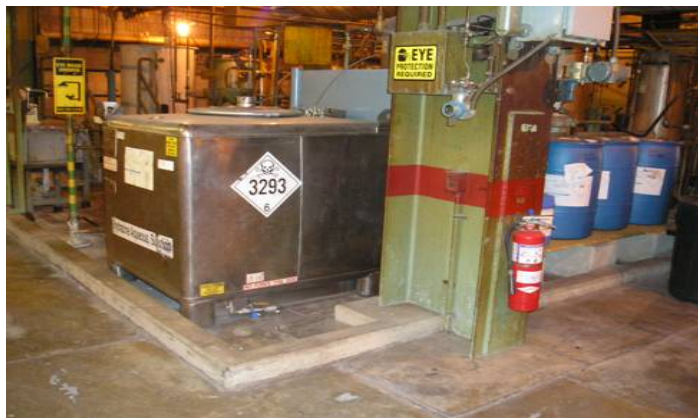
Figure 7. Hydrazine area at the time of the initial audit visit. The metal tote is on the left.
