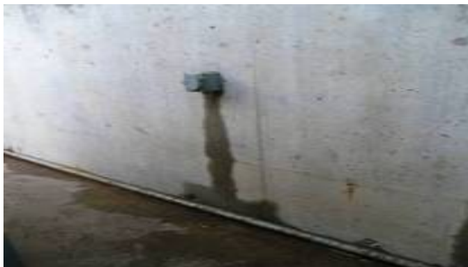
Figure 12. Water leaked through an electrical box.
