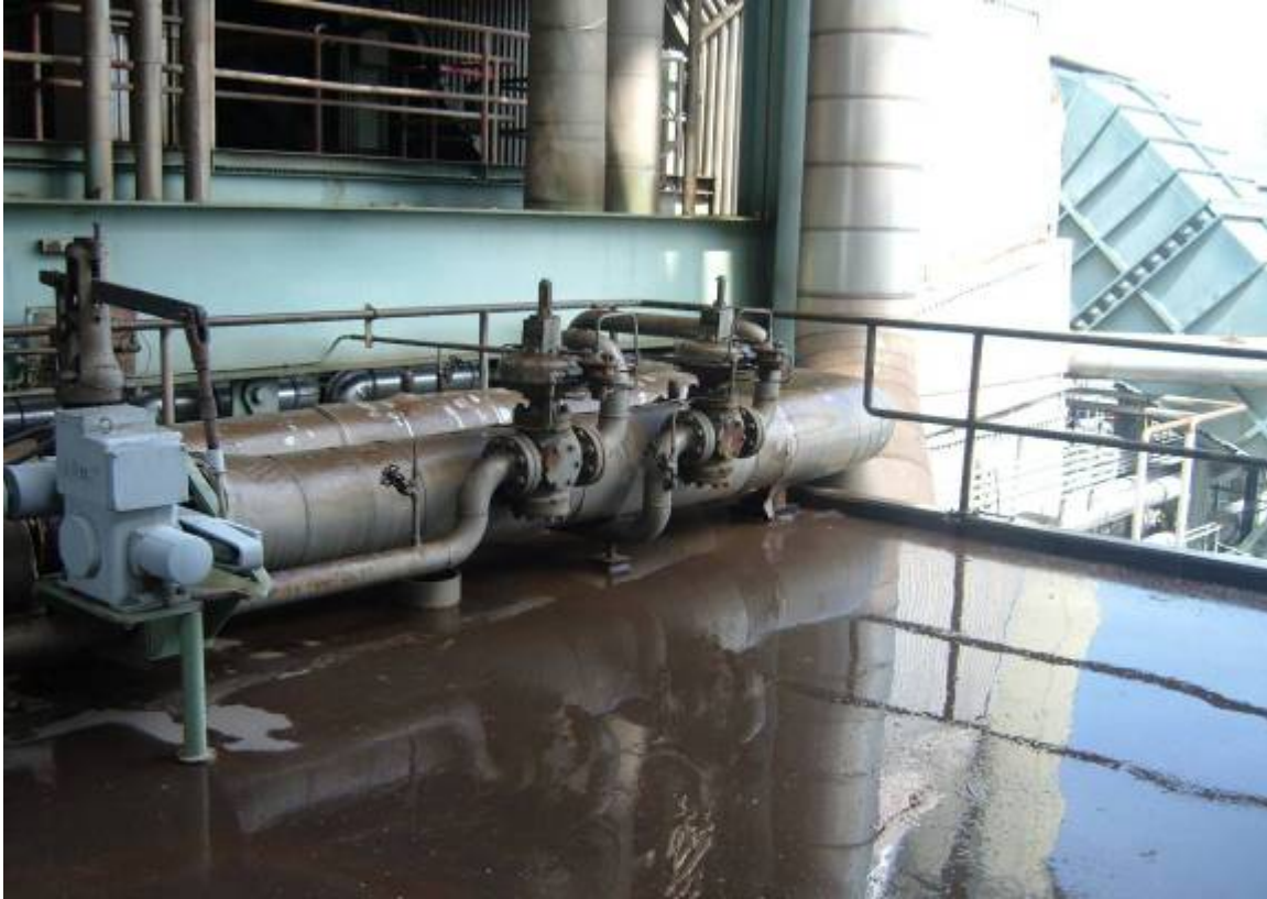
Figure 1. Water creates hazard in walkway.
