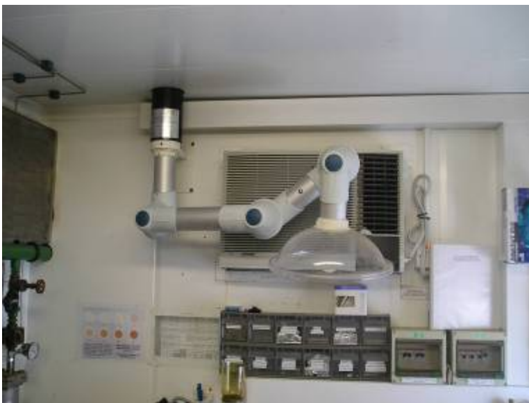
Figure 13. The Units 1 and 2 boiler chemistry lab contains a fume hood.
