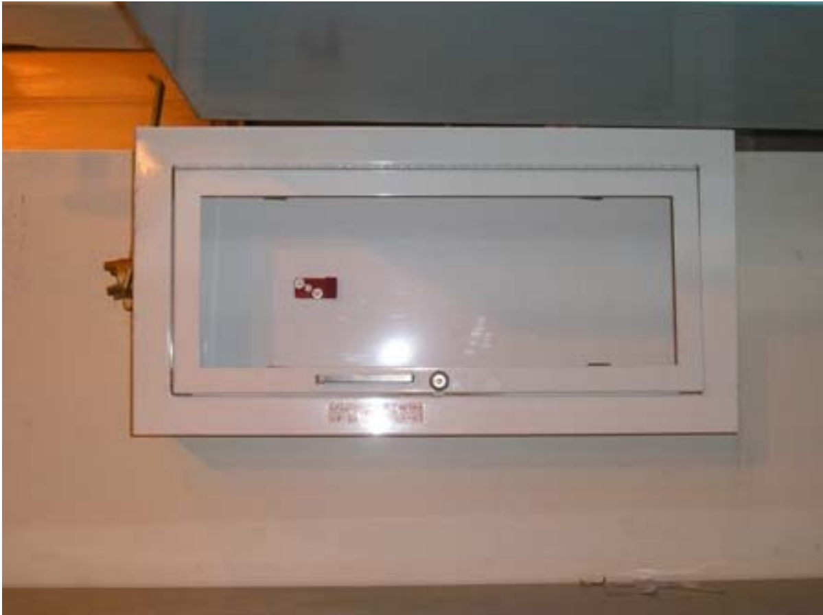
Figure 8. Cabinet is missing a fire extinguisher.
