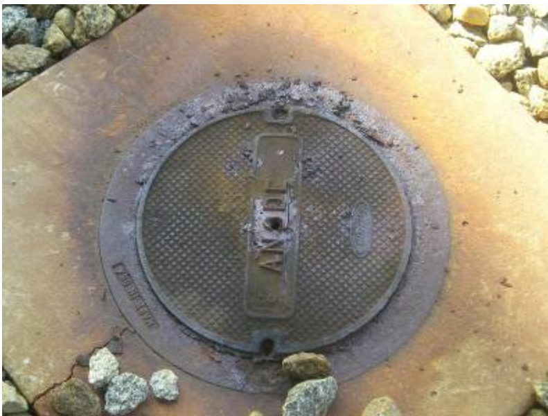
Figure 10. These anodes for the impressed current cathodic protection system corrode as they deliver a current to protect piping.
