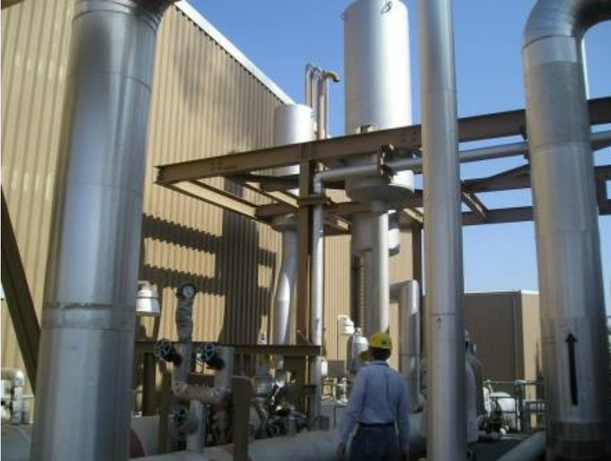
Figure 9. Handwritten direction arrows on piping indicate the need for better labeling.
