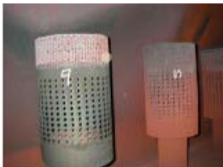
Figure 15. Enlarged holes indicate some FAC on steam separator cans. 51
