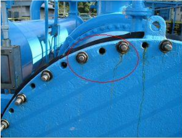
Figure 1: Bearing cooling water heat exchanger is missing 50% of the endplate bolts and nuts.
