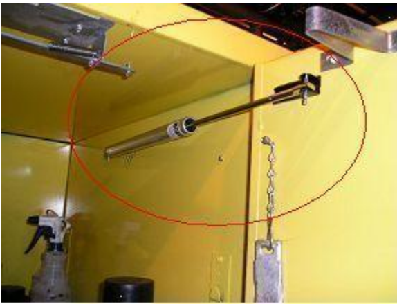
Figure 8: Flammable cabinet with self-closers
