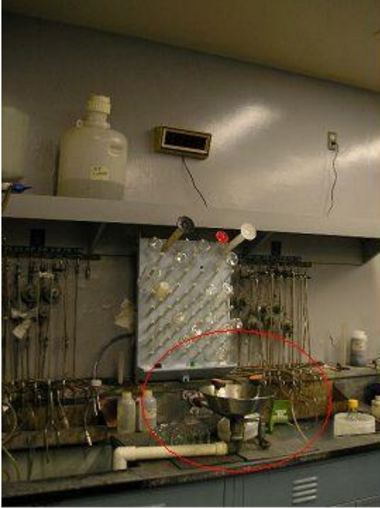
Figure 7: Eye wash station with no emergency shower overhead.
