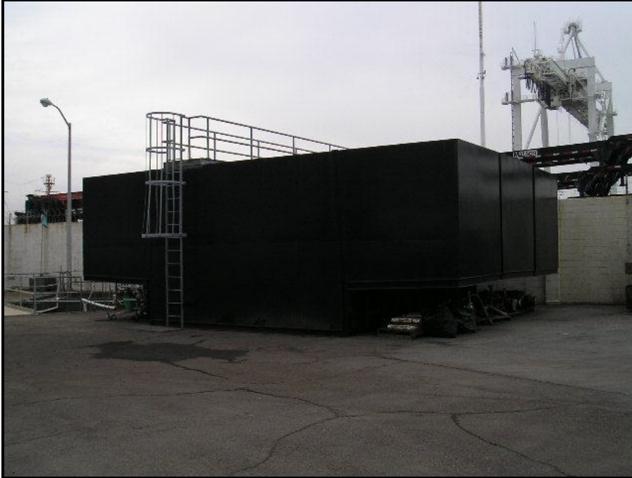
Figure 3 -- This “Baker” tank is not reflected on the Facility Layout/Drainage Map.
