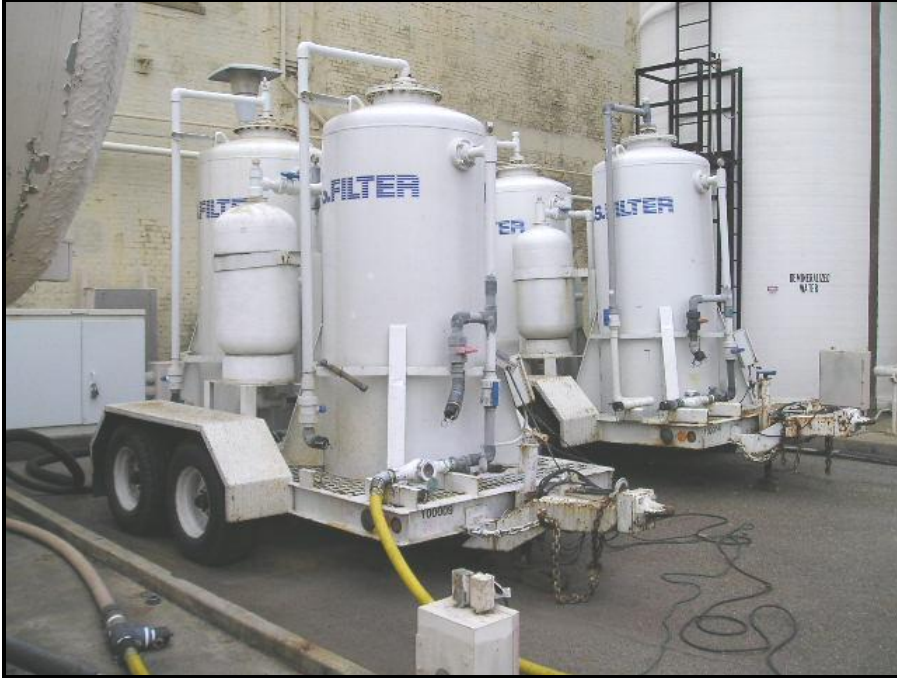
Figure 2 -- Existing mobile demineralizer tanks.
