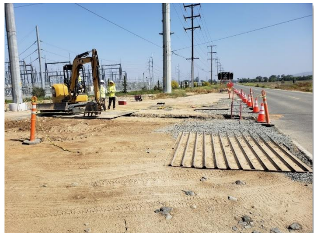
Figure 14. Unstabilized construction entrance on west side of Menifee Road near the underground trenching
