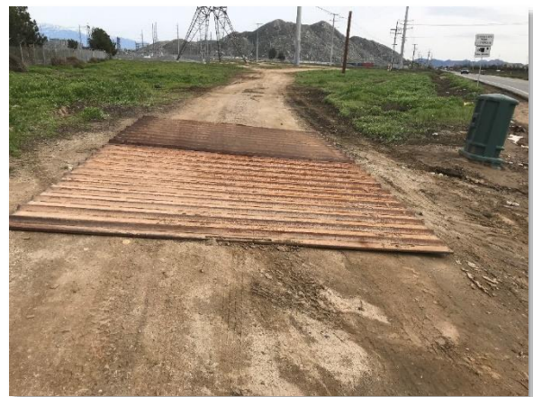
Figure 2. Shaker plate for track-out control was delivered to the Valley Substation Yard driveway.
