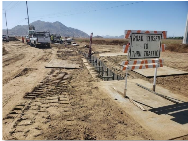
Figure 10. Placing conduit in the trench from Menifee Road to Construction Area UNK250
