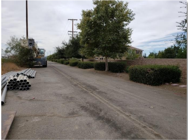
Figure 13. Uncapped pipes and a piece of construction equipment staged without secondary containment near UNK222
