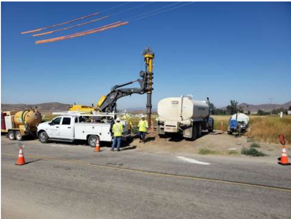
Photo 2 – Foundation drilling at Construction Area UNK20 with traffic control in place on Leon Road (June 10, 2019).
