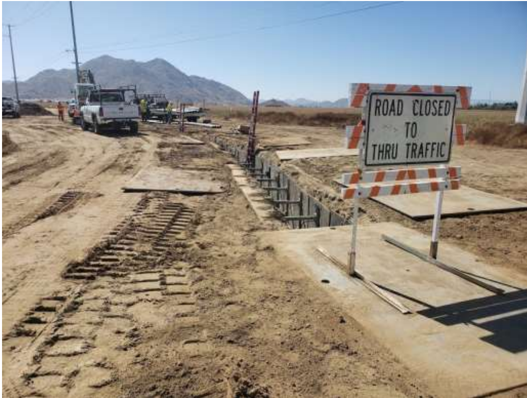
Photo 3 – Placing conduit in the trench from Menifee Road to Construction Area UNK250 (June 17, 2019).
