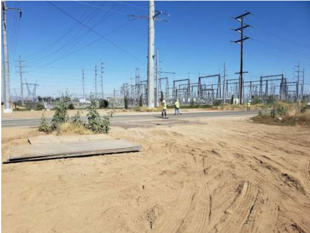
Photo 4 – Construction crew sweeping track out off of Menifee Road from the unstabilized entrance on the east side of Menifee Road (July 17, 2019).
