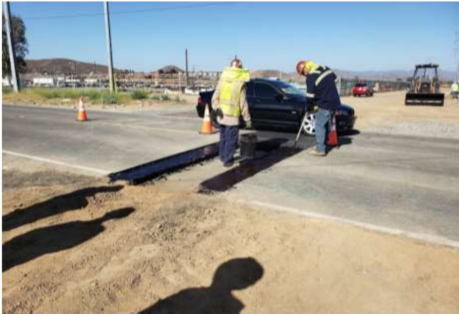
Photo 1 – Paving activities on Menifee Road for the northern underground section near Valley Substation (July 24, 2019).
