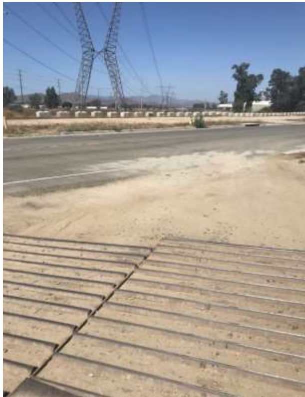
Photo 2 – Track-out at the construction entrance without proper SWPPP TC-1 required stabilization off Matthews Road to the Valley Yard (July 24, 2019).
