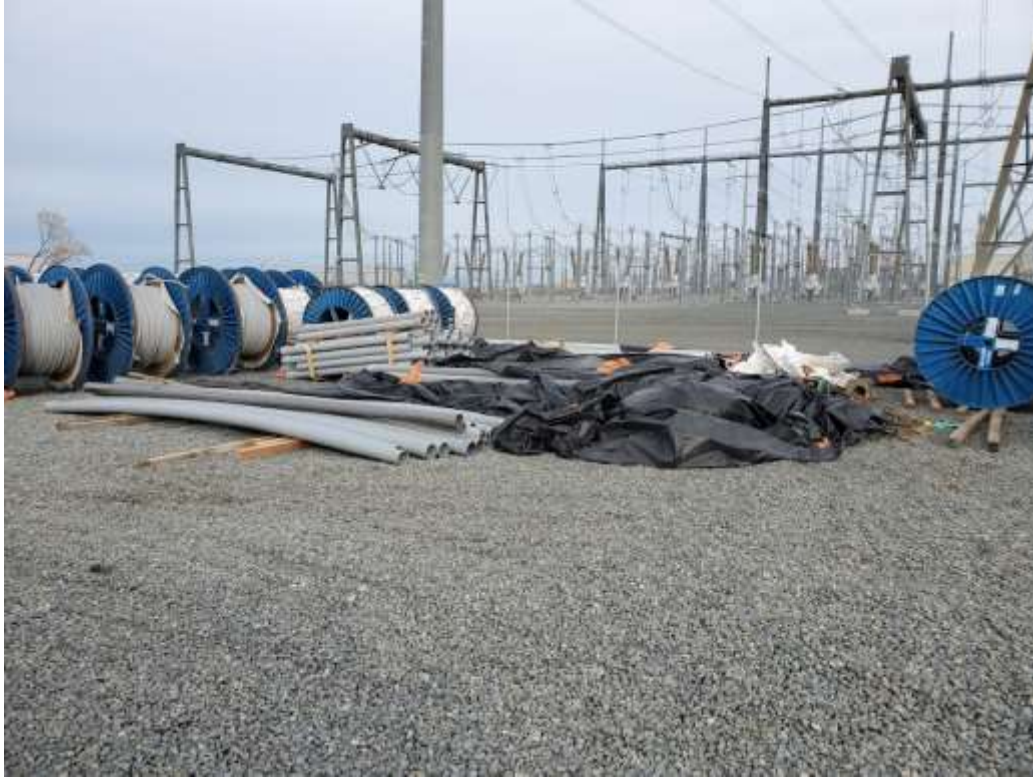
Photo 3 - Uncovered pipes at Valley Substation Yard (December 3, 2019).
