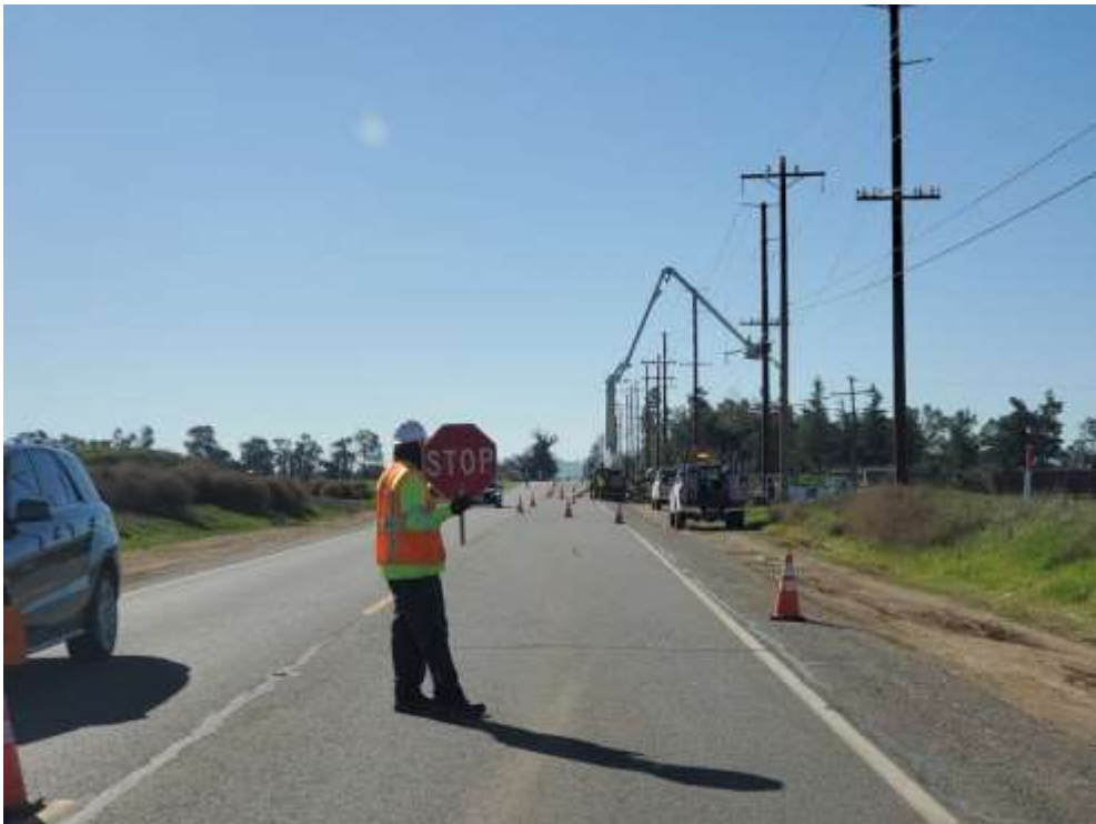
Photo 4 – Traffic control in place during distribution wire stringing for Construction Areas UNK155 through UNK191 (January 28, 2020).
