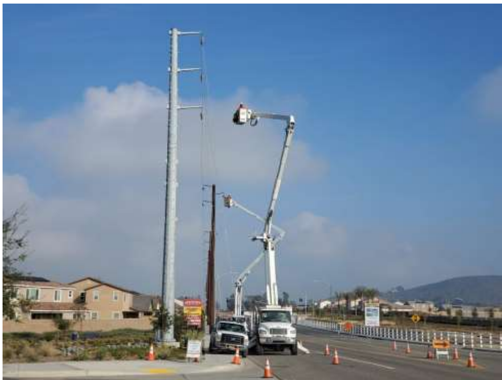
Photo 2 – Wire stringing activities at Construction Areas UNK206 with traffic control in place (January 22, 2020).
