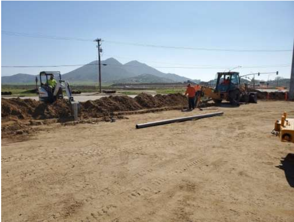
Photo 5 – Trenching outside approved project disturbance area limits between Construction Areas UNK44 and UNK45 (February 19, 2020).
