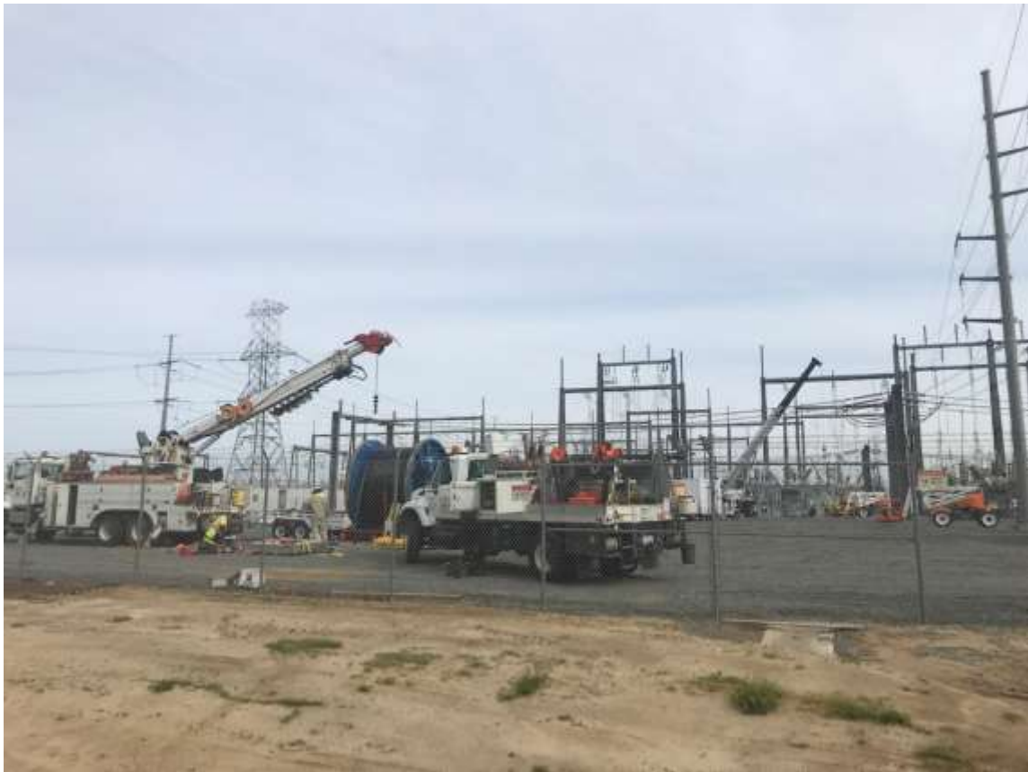
Photo 3 – Pulling cable at the underground vault within the Valley Substation (March 31, 2020) (Photo courtesy of SCE).
