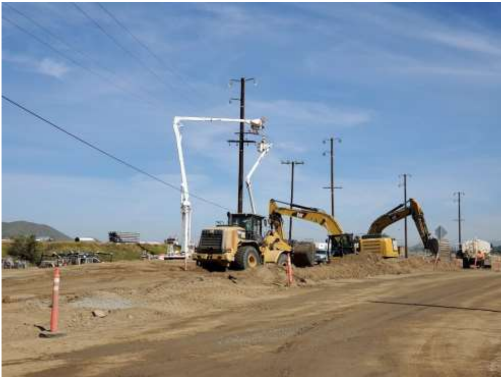
Photo 2 – Wire stringing activities at Construction Area UNK54. Please note that ground disturbing construction activities in the foreground of photo is non-project related. (May 6, 2020).
