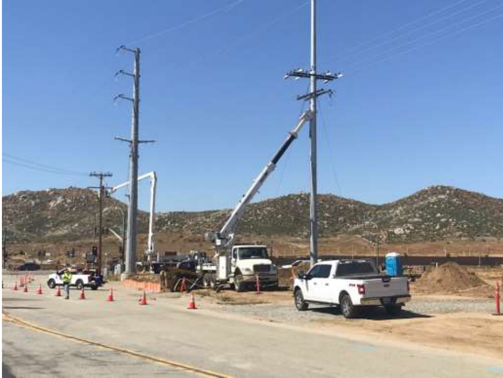
Photo 3 – Underground trenching activities at Construction Area UNK44 to UNK45 (May 22, 2020) (Photo courtesy of SCE).
