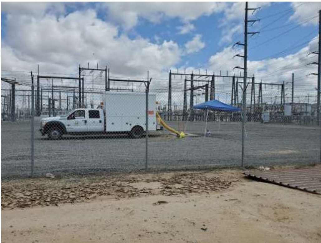
Photo 4 – SCE crews working in vault inside Valley Substation (May 13, 2020).
