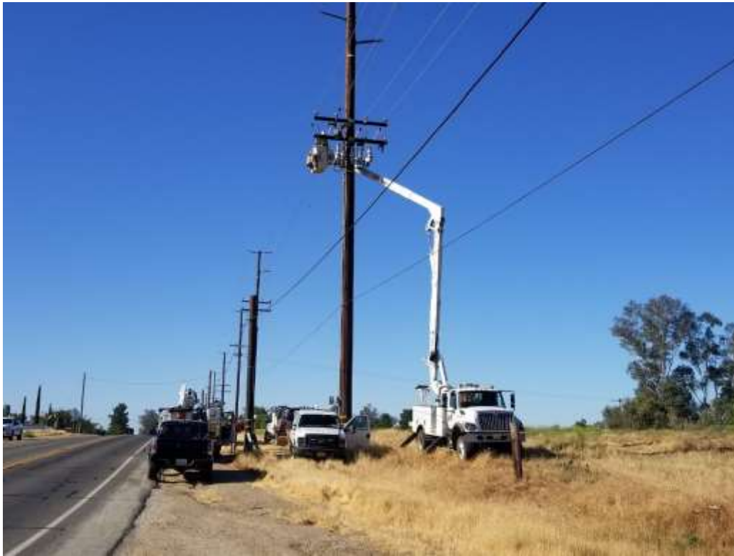
Photo 3 – Capacitor bank energization activities at Construction Area UNK156 (May 27, 2020) (Photo courtesy of SCE).
