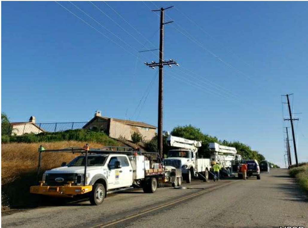
Photo 1 – Guy wire attachment replacement at pole 4937033E (June 26, 2020) (Photo courtesy of SCE).
