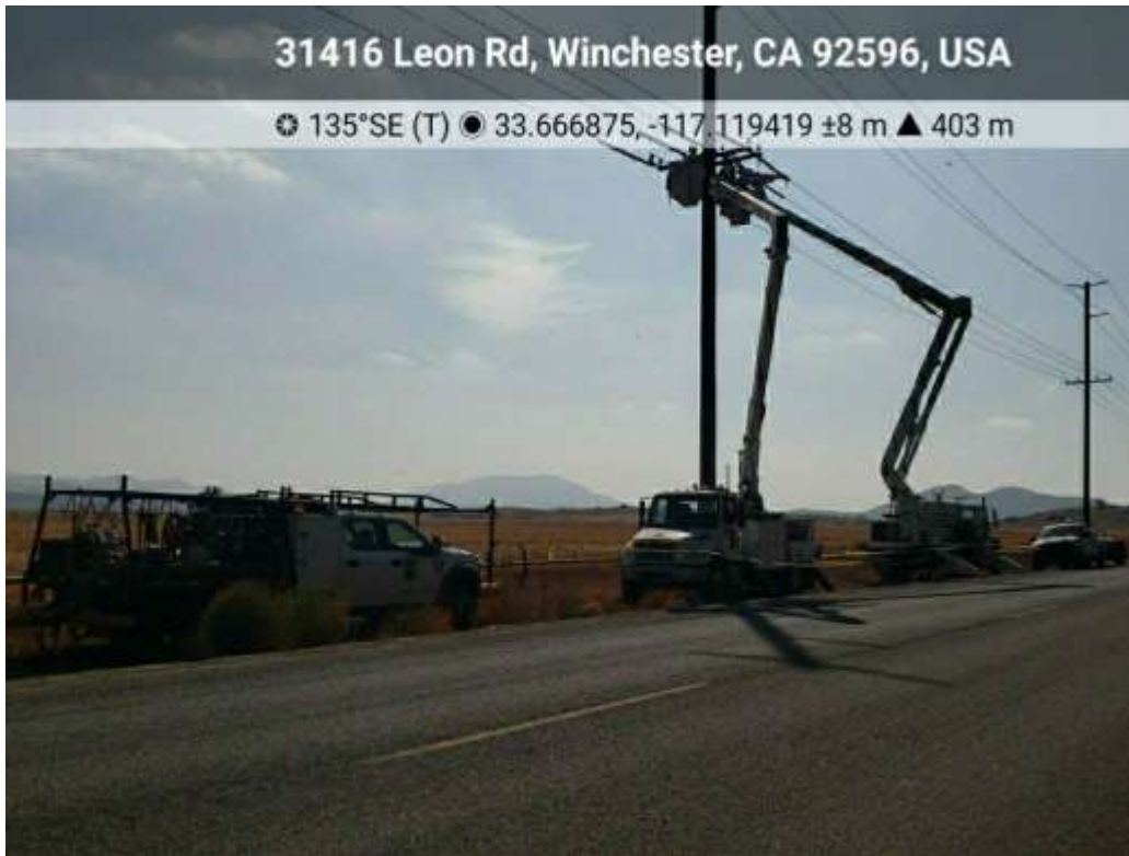
Photo 1 – Dead end installation at Distribution Pole 4936675E (October 22, 2020) (Photo courtesy of SCE).
