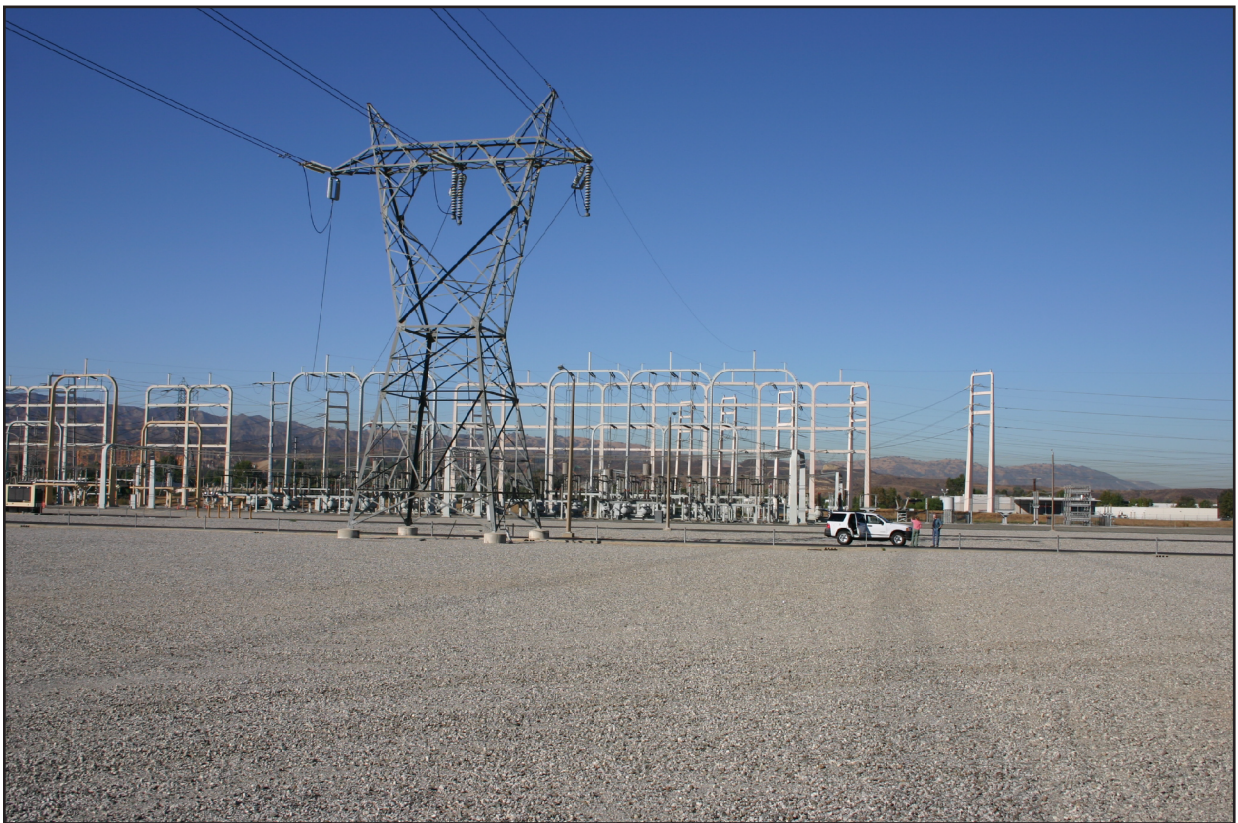
13 Existing transmission line entering Pardee Substation.
