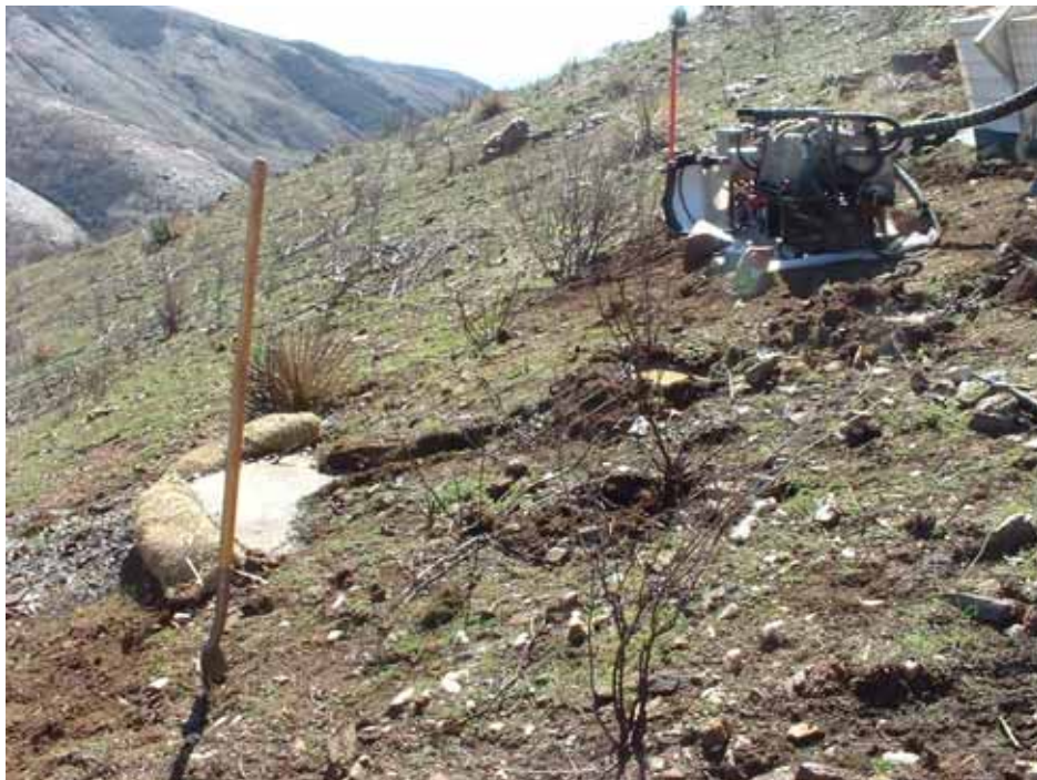
Figure 2: Straw wattles and catchment basins used to contain drilling mud at geo-tech sites at Tower site 53.
