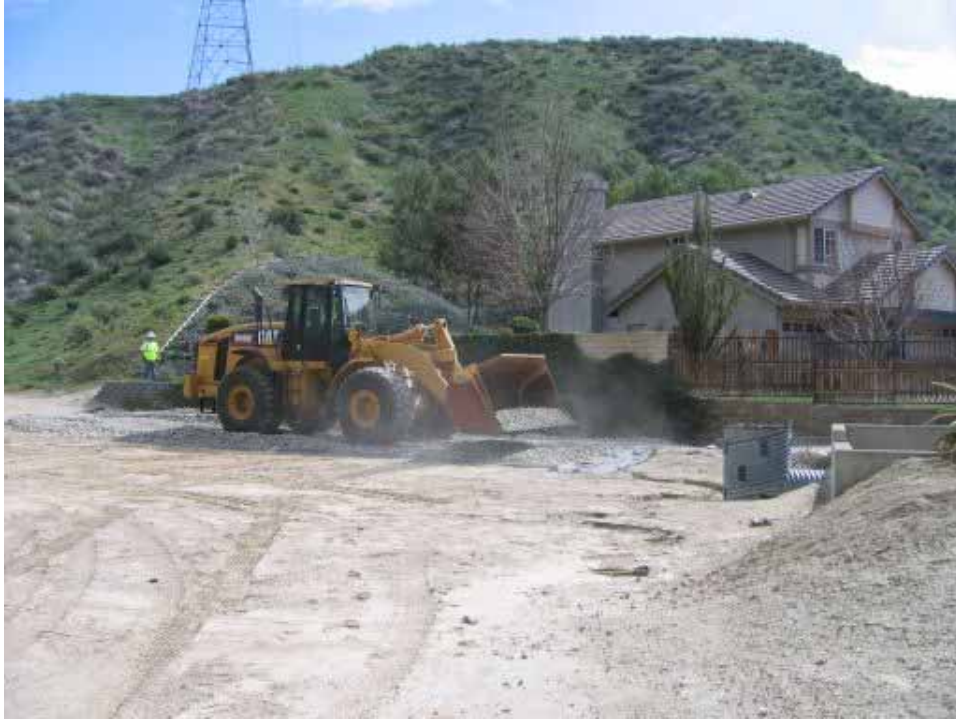
Figure 1: Rock was placed where the Shoofly access meets public roads in order to minimize dirt tracking outside of the right-of-way.
