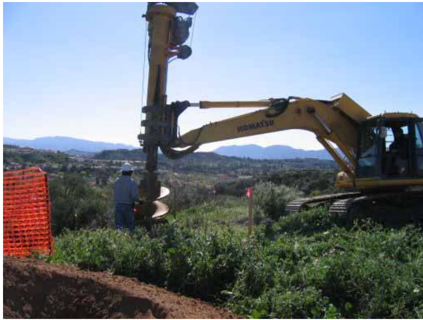
Figure 3: After the road crew prepares the access to the Shoofly tower site, the drilling crew mobilizes and drills the pole structure foundation holes.
