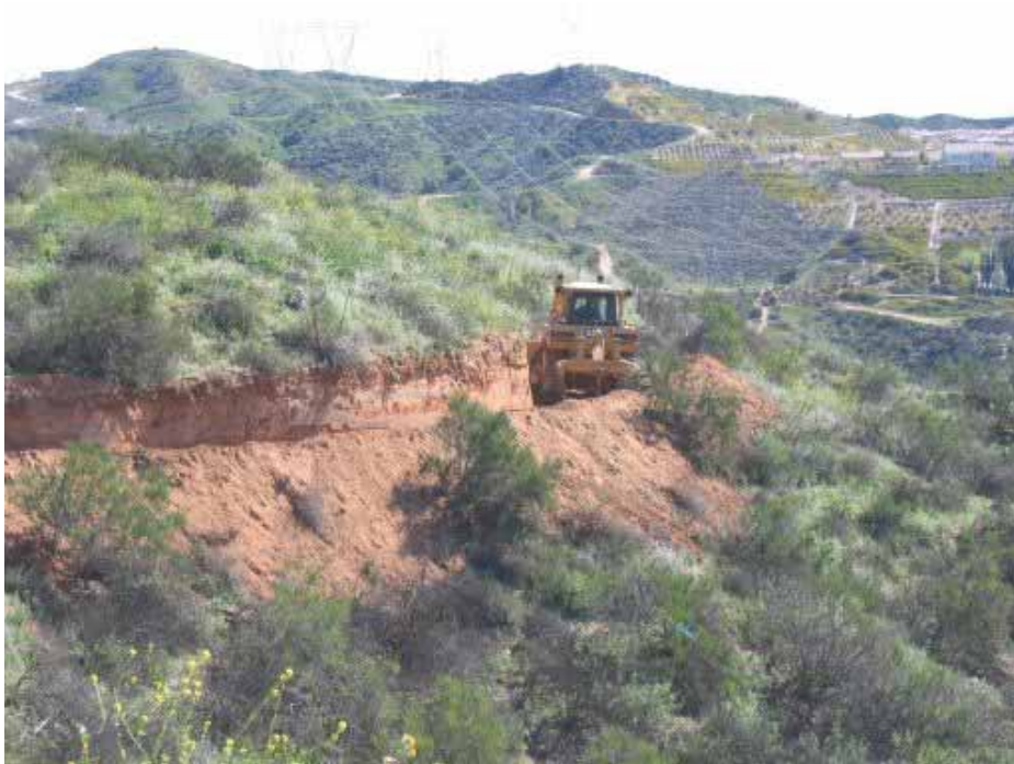
Figure 2: New temporary roads were constructed to Shoofly structure 2. Silt fencing was installed below the loose material to prevent erosion into adjacent areas.
