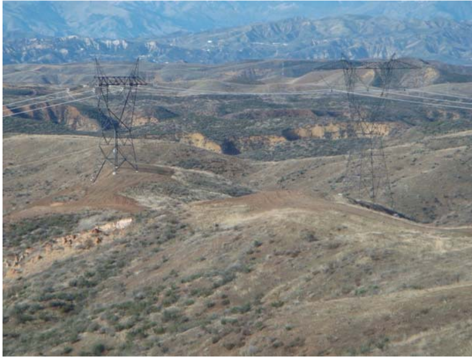
Figure 1: Restoration of ANF access road between Towers 33 and 34, Segment 1. Seeding has already taken place using the imprinting method.
