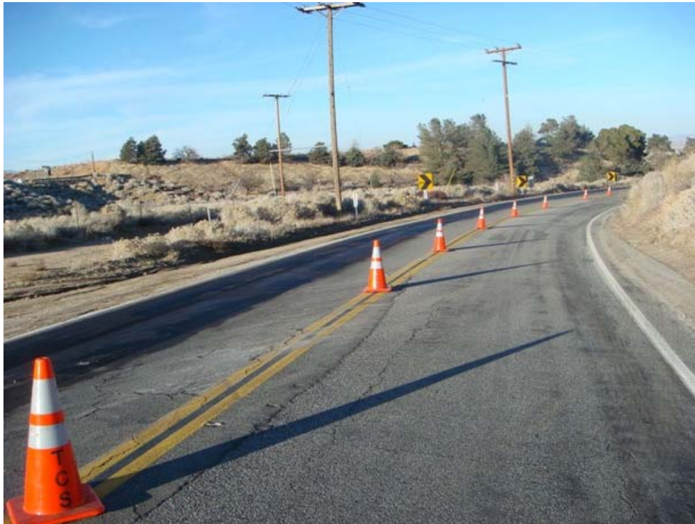
Figure 2: Road repair along Johnson Road near 110 th Street in Section 3, Segment 1. Construction crews caused damage to the pavement when moving equipment in the summer of 2008.
