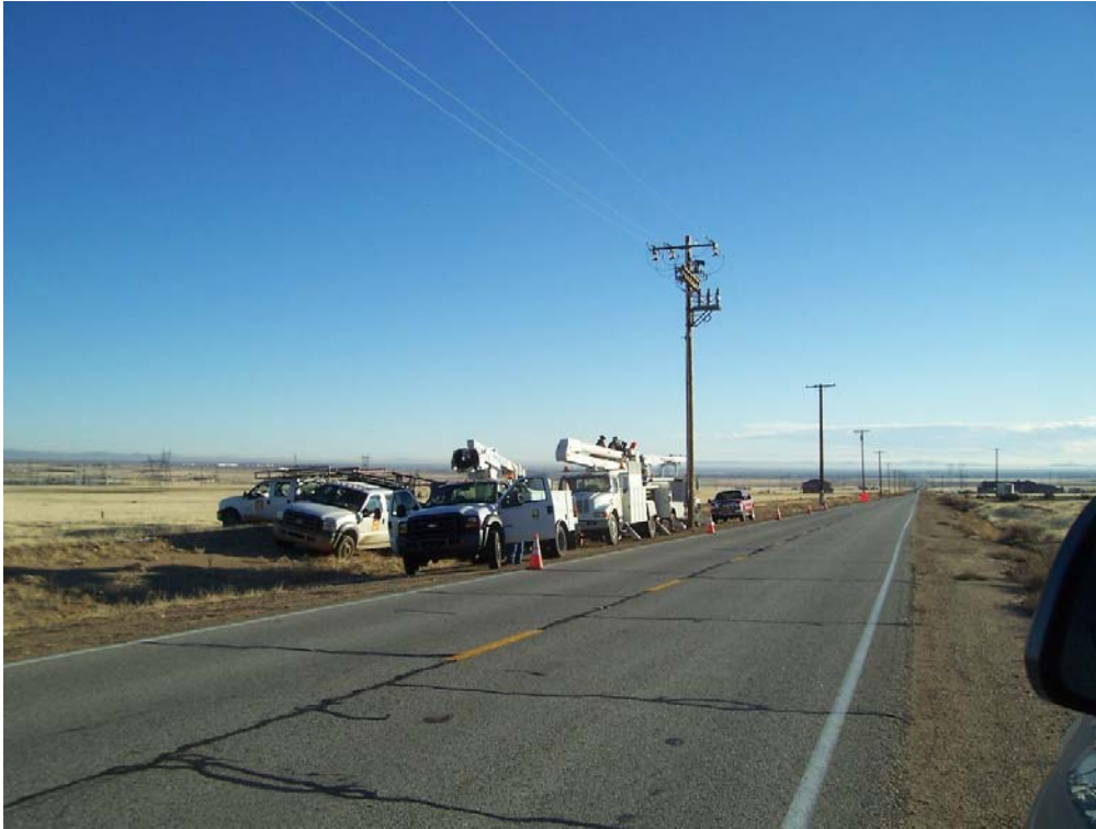
Figure 1: Auto Recall Riser Relocation, 12 kV Lake Hughes Line.
