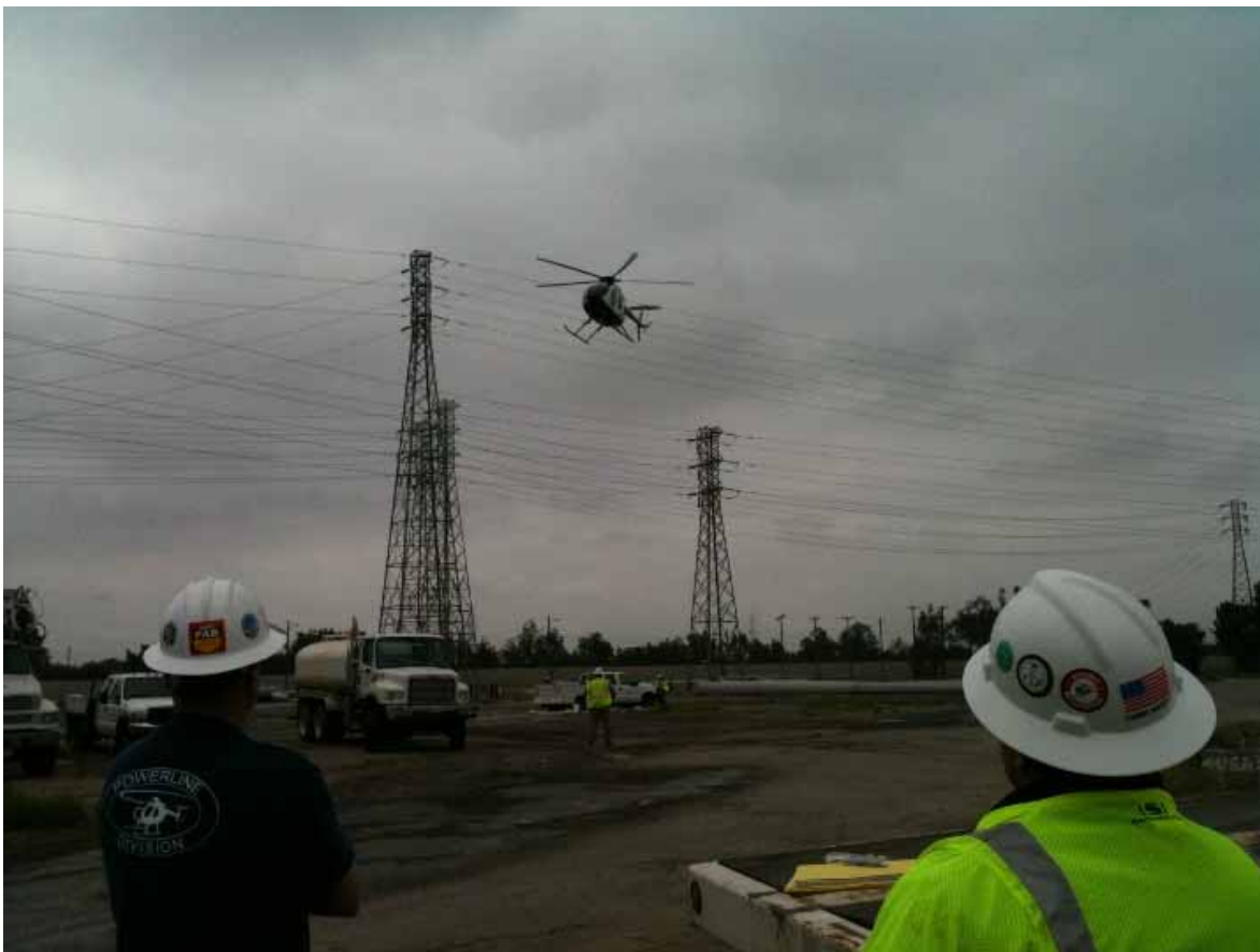
Figure 4: Helicopter installation of the Segment 7 Telecom line near the Rio Hondo Substation.
