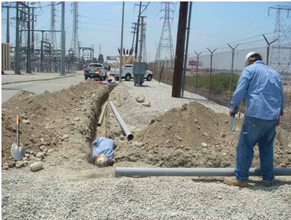
Figure 3: Trenching inside of the Rio Hondo Substation for the Segment 7 Telecom work.
