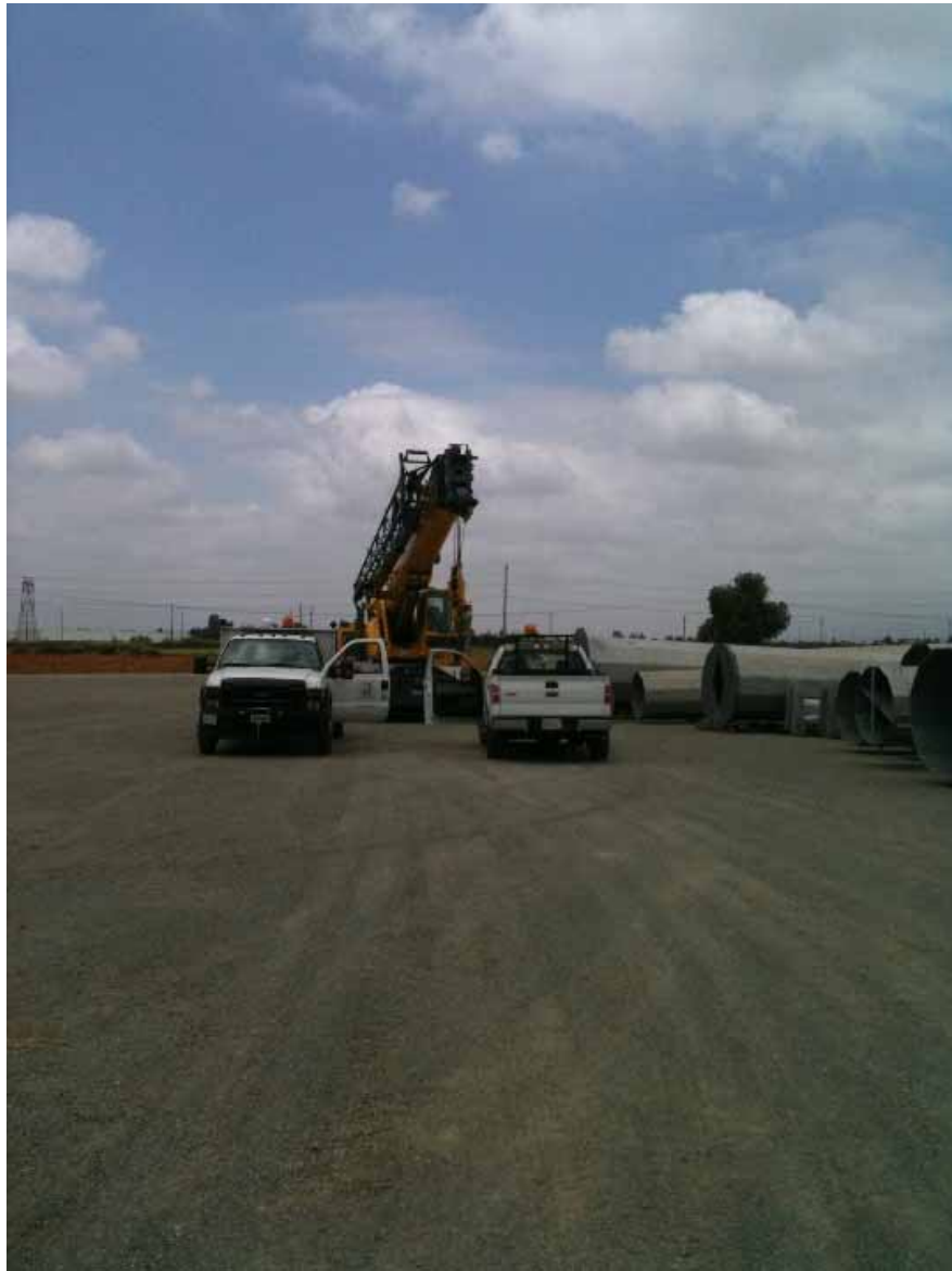
Figure 2: Material delivery to the Rancho Vista Yard. Exclusion fencing for the Delhi sands flower-loving fly area is seen in background.
