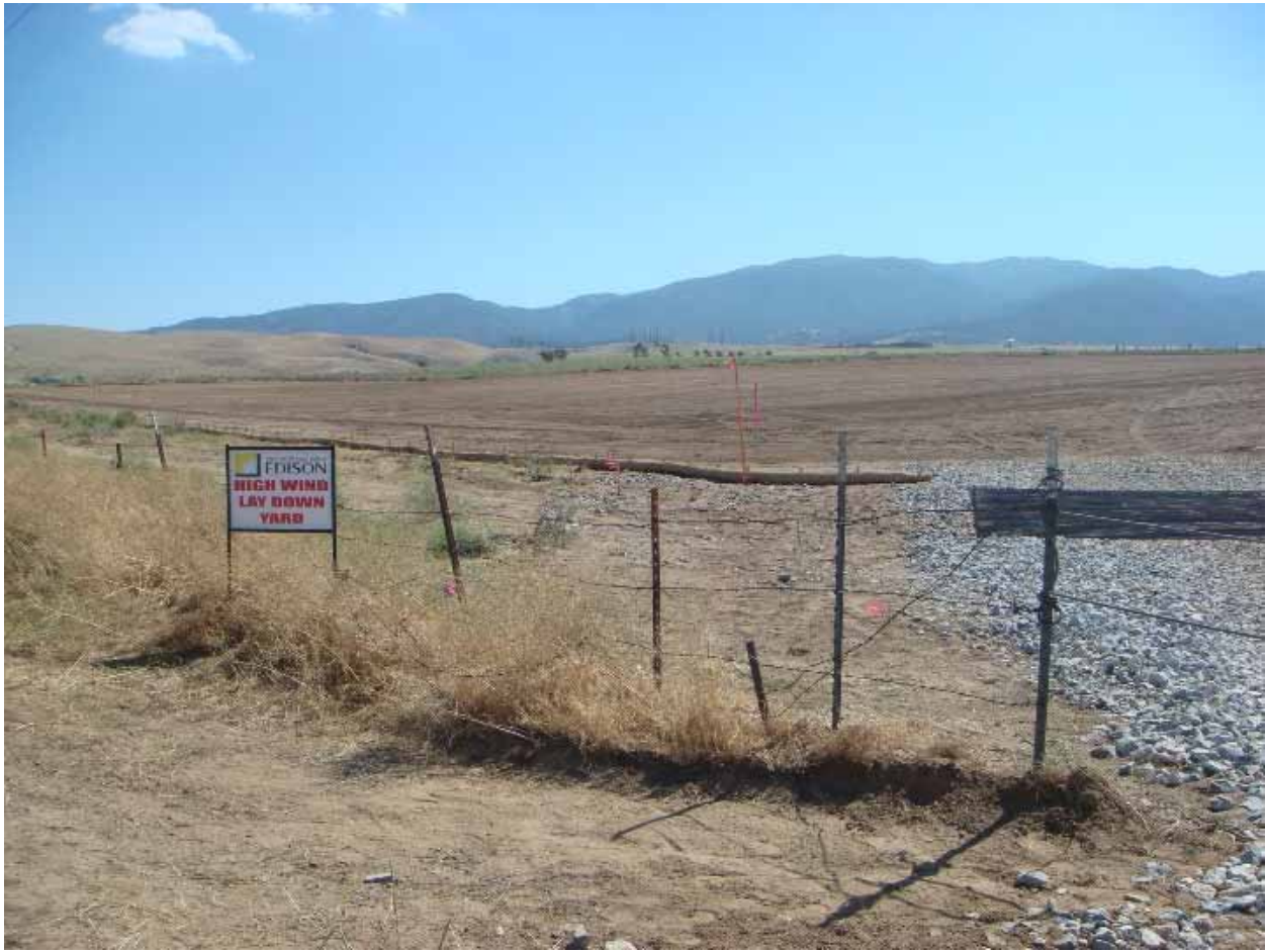
Figure 2: Construction of the new Highwind Material Yard near the site of the future Highwind Substation in Tehachapi.
