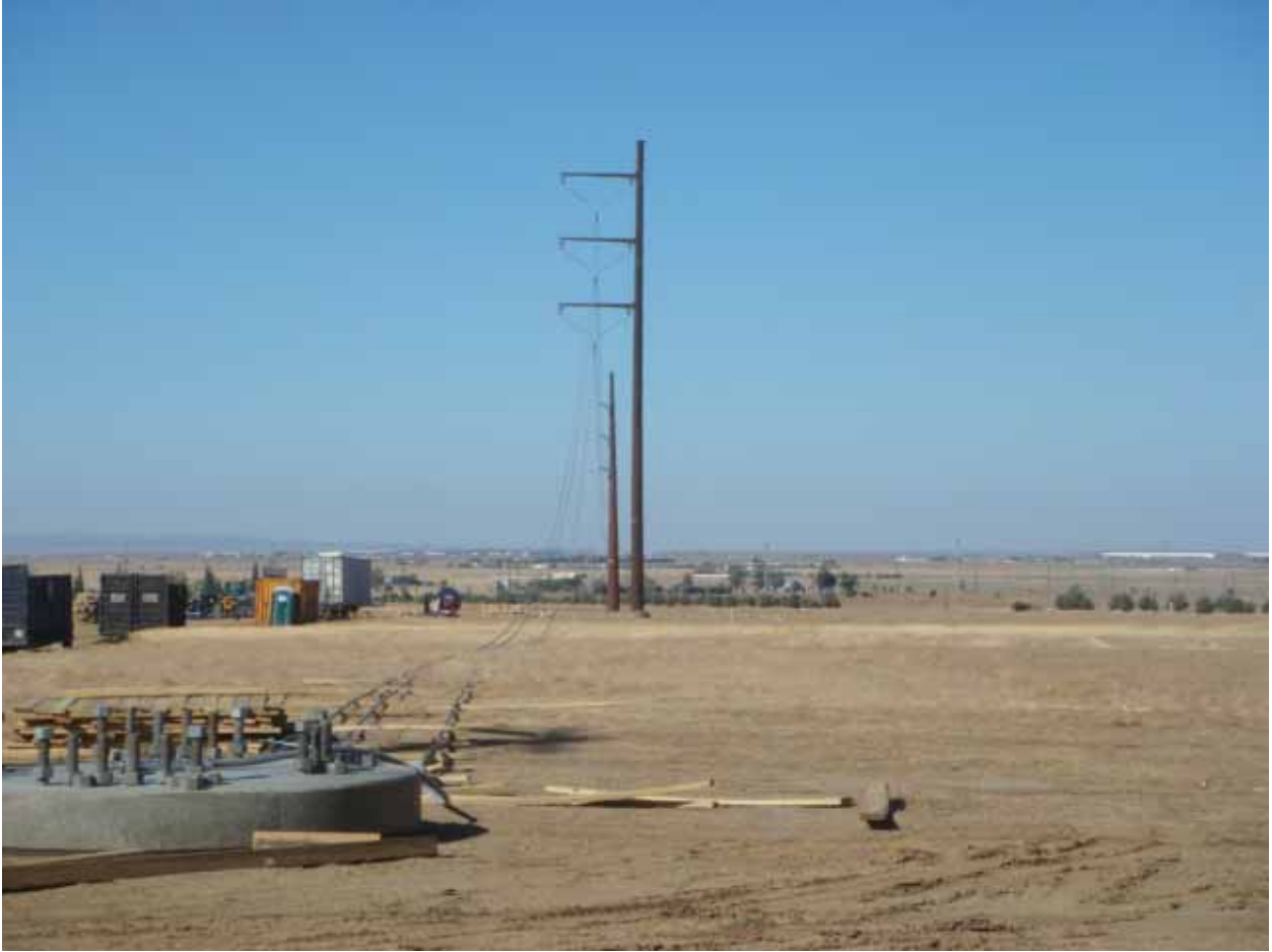
Figure 1: Stringing of the relocated Sagebrush 220 kV line surrounding the Antelope Substation expansion area.
