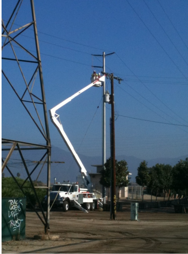
Figure 3: 66 kV crews working on the Rio Hondo-Amador-Jose-Mesa Line install wire on a new pole in a nursery in Baldwin Park.
