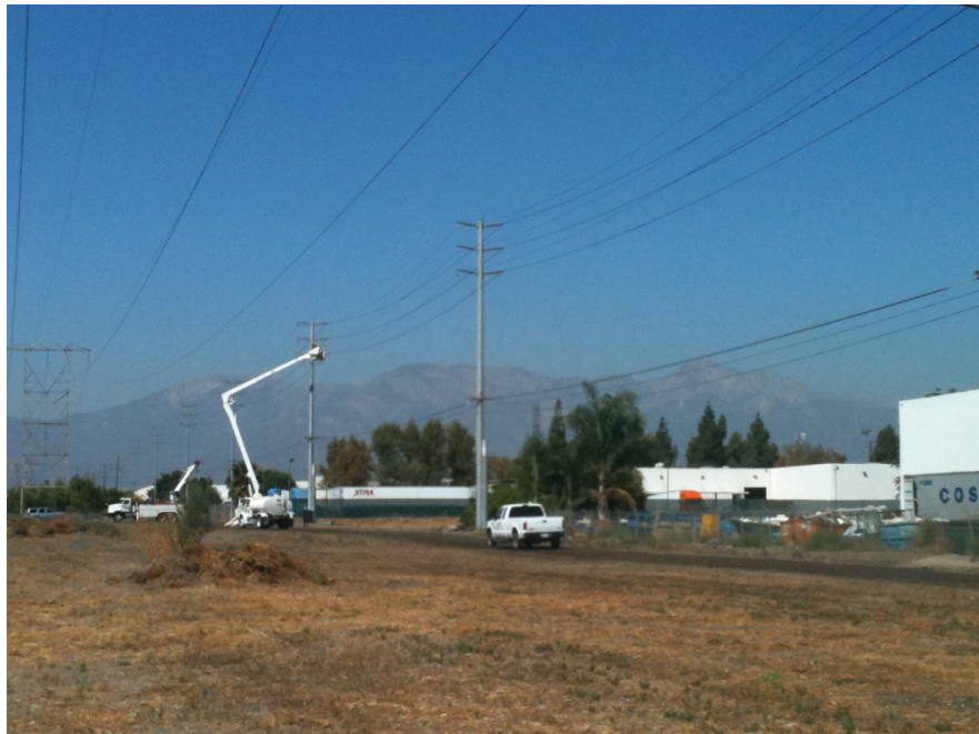
Figure 4: 66 kV crews working on the Chino Substation relocation line between Eucalyptus Avenue and Chino Hills Parkway.
