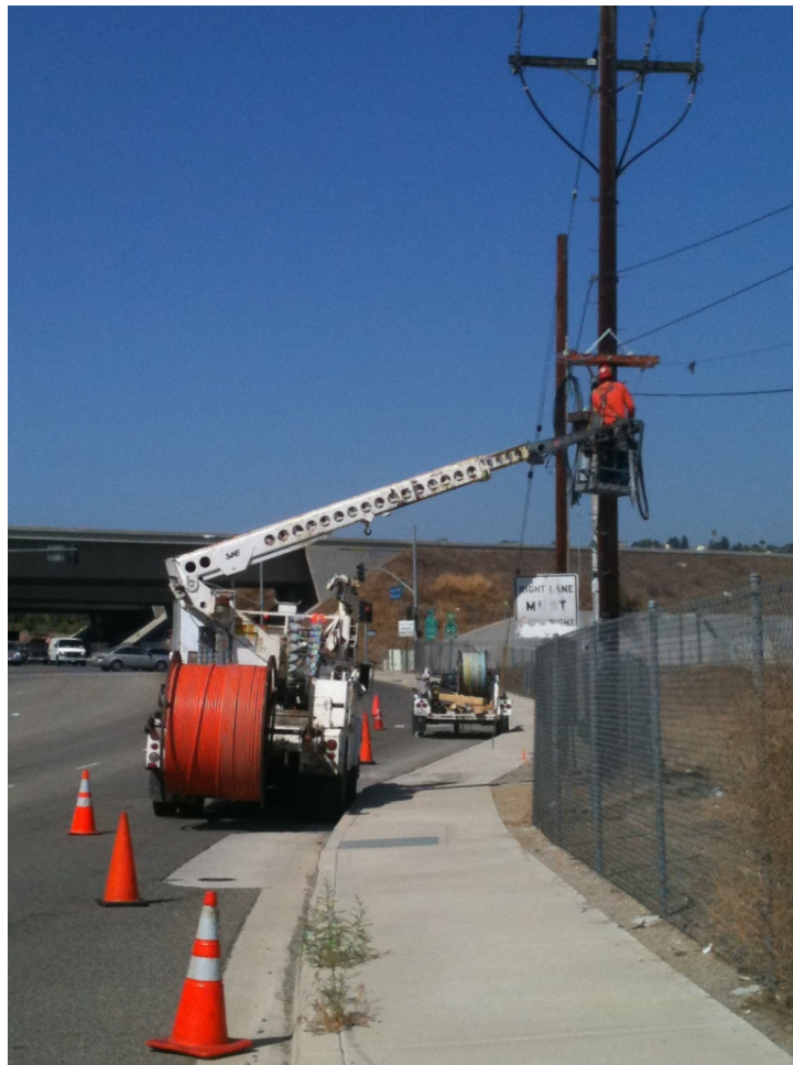
Figure 5: A Segment 8 Telecom aerial crew installs fiber optic cable on Chino Avenue adjacent to the 71 Freeway.
