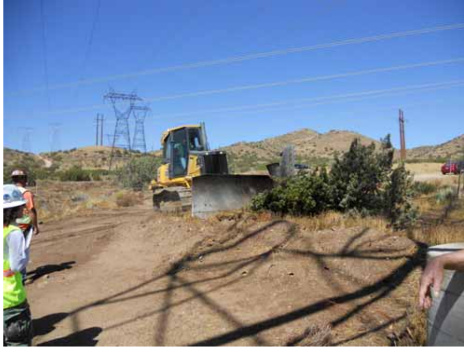
Figure 3: Tree removal at Tower 61 on Segment 5. The Juniper trees were evaluated for potential bat roosts prior to removal.
