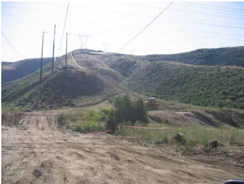
Figure 2: An Environmentally Sensitive Area (ESA) shown surrounded by pink flagging, was encroached upon during wire stringing between Shoofly poles 13 and 14. The wire seen above entered the ESA and hit the elderberry tree containing two bird nests. No biological monitor was present during the work in this location.
