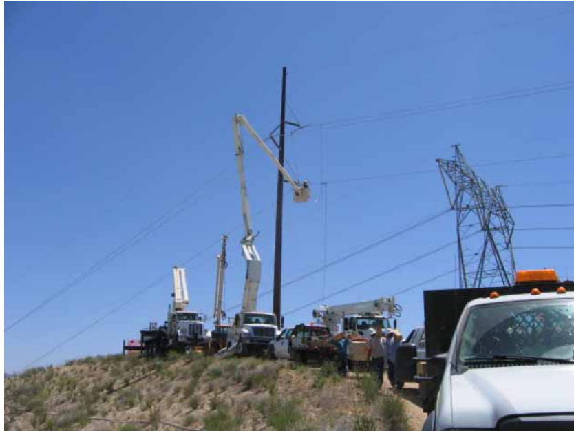
Figure 1: The relocation of Shoofly pole 9, due to low ground clearance of the wire. The wire was already strung in, but was unclipped and supported during the pole relocation.
