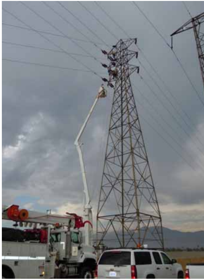
Figure 3: On the Rio Hondo–Amador-Jose-Mesa 66 kV line, crews rearrange a line connection on a tower north of Ramona Boulevard.
