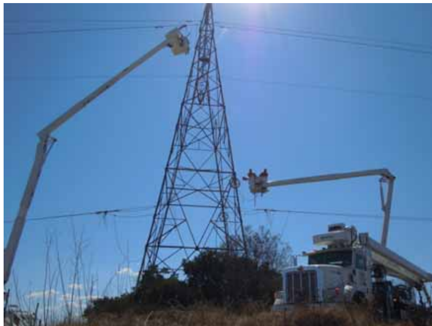
Figure 4: In Tonner Canyon, crews install travelers on old transmission lines prior to removal.
