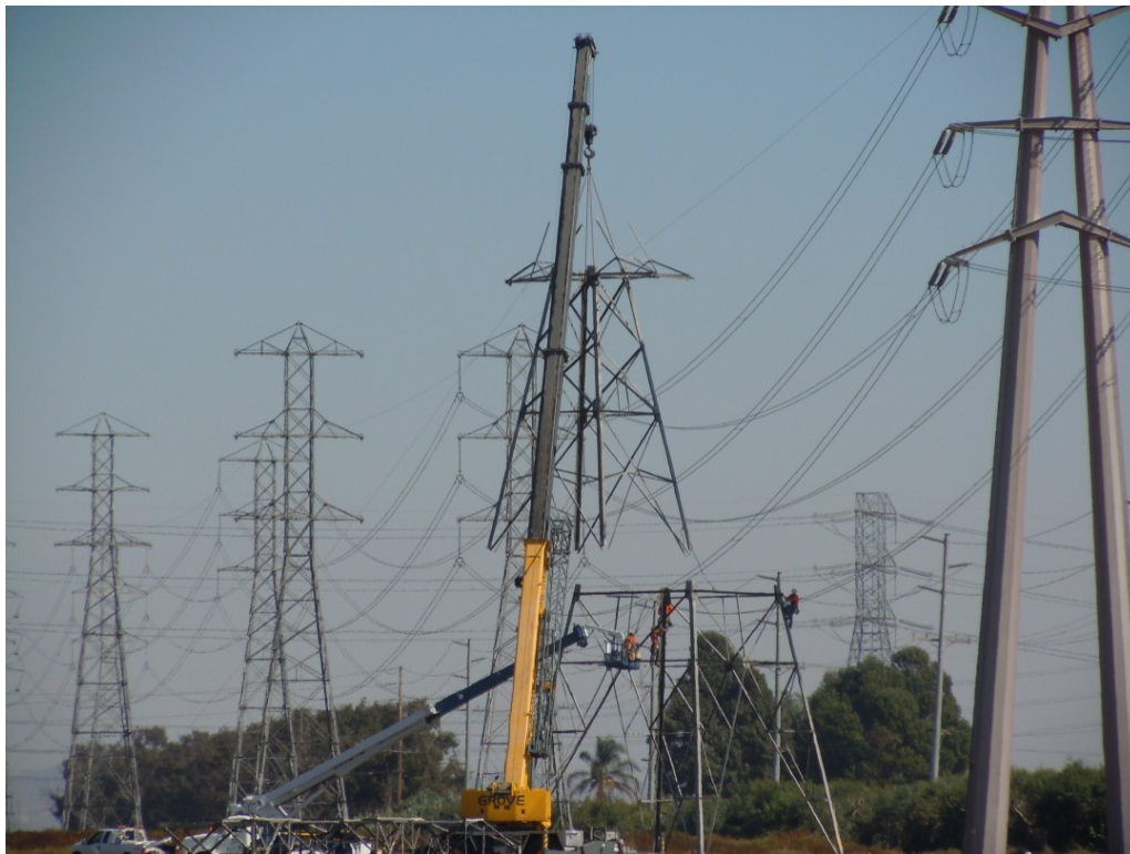
Figure 4: In the City of Ontario, Wilson crews work to remove a tower, Segment 8 Phase 2.
