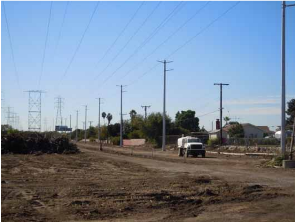
Figure 3: Newly installed Rio-Hondo-Amador-Jose-Mesa 66 kV poles within Gallos Nursery in the City of El Monte.
