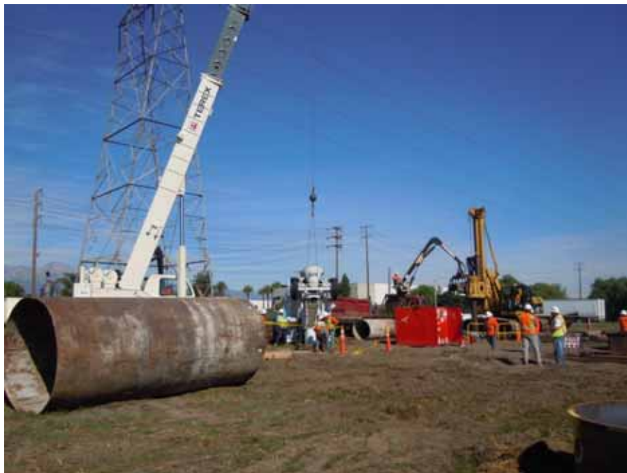
Figure 6: Segment 8 Phase 2, concrete pour for Tower M0-T3 foundations, outside of Chino Substation.
