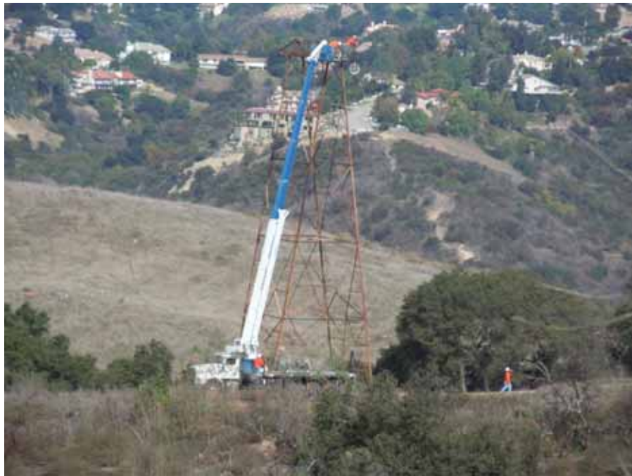
Figure 5: A Wilson lineman removes a traveler in preparation for tower wreck-out in Tonner Canyon, Segment 8, Phase 1.
