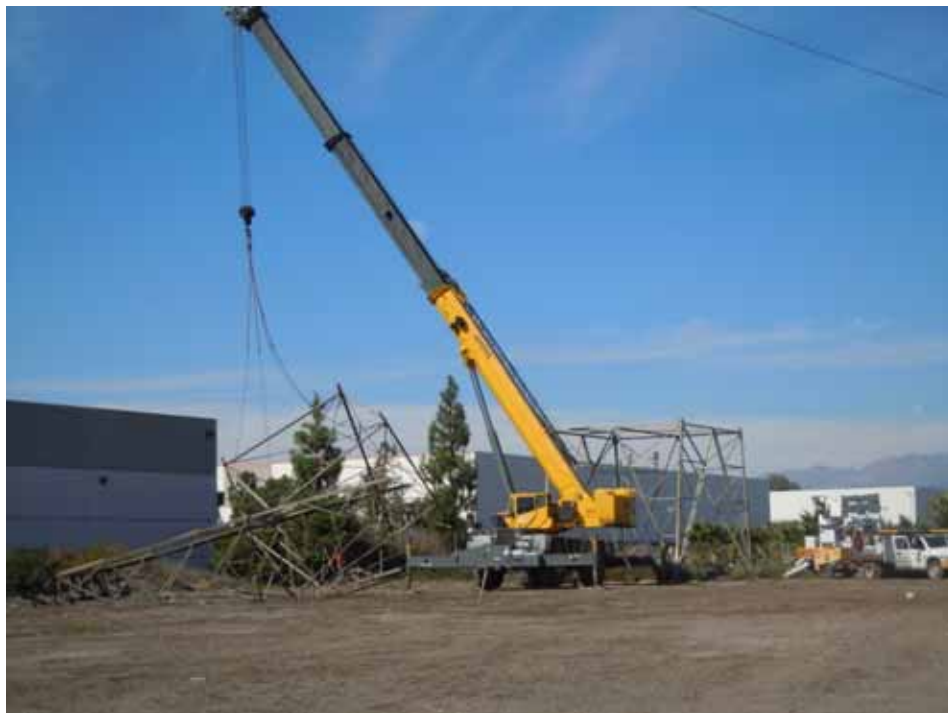
Figure 4: A Wilson crew works to remove Tower M66-T2 in the City of Chino, Segment 8, Phase 2.
