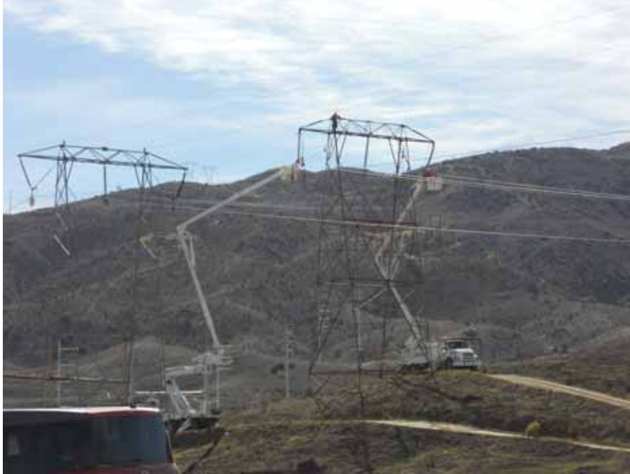
Figure 1: Segment 5: Wire removal from existing 220 kV lines during the Sagebrush Transmission Line outage near Tower 37.
