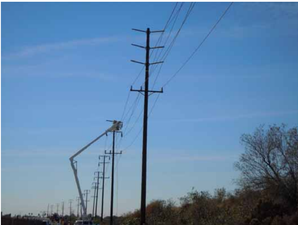
Figure 4: An SCE crew re-conditions a pole on the Rio Hondo–Amador 66 kV line in the City of Irwindale.
