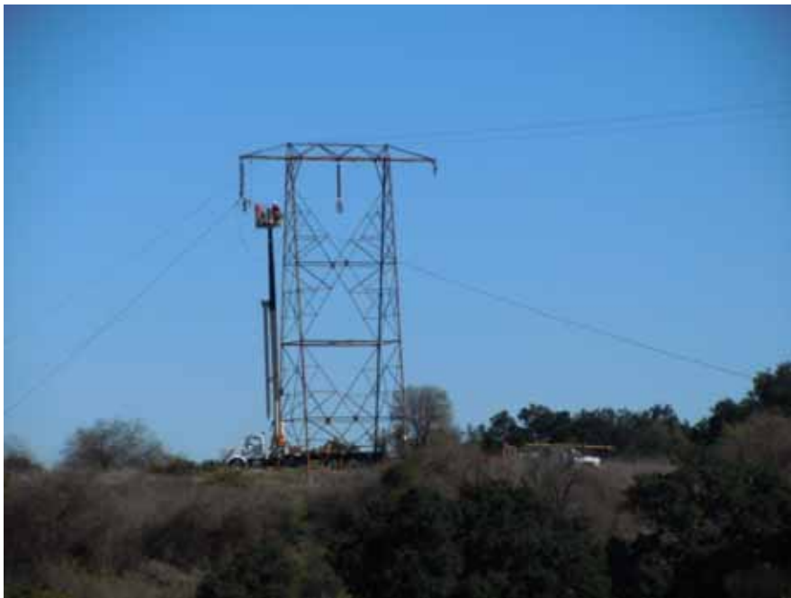
Figure 6: A Wilson crew removes wire at Tower M58-T3 in Tonner Canyon, Segment 8, Phase 1.
