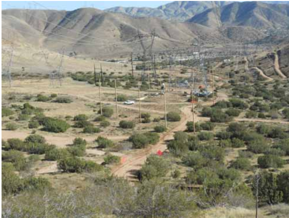
Figure 2: View of guard pole structures between Towers 60 & 61 in preparation for wire removal from existing 220 kV wreck-outs, Segment 5.
