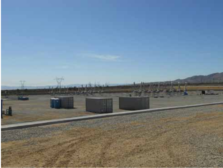
Figure 1: View of circuit breakers in Windhub Substation.
