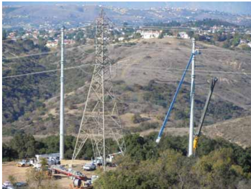
Figure 4: An SCE crew strings wire on the Shoofly at Tower M57-T3, Segment 8 Phase 1.
