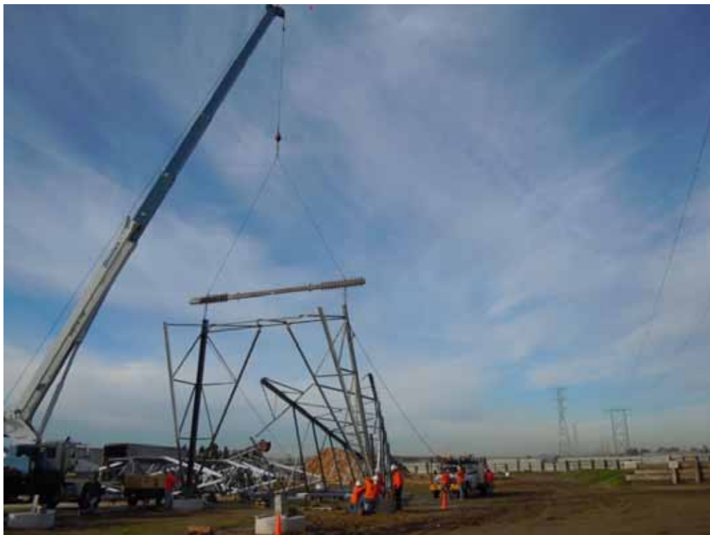
Figure 4: A Wilson crew assembles Tower M4-T in Ontario, Segment 8, Phase 2. Newly erected towers are visible in the background.
