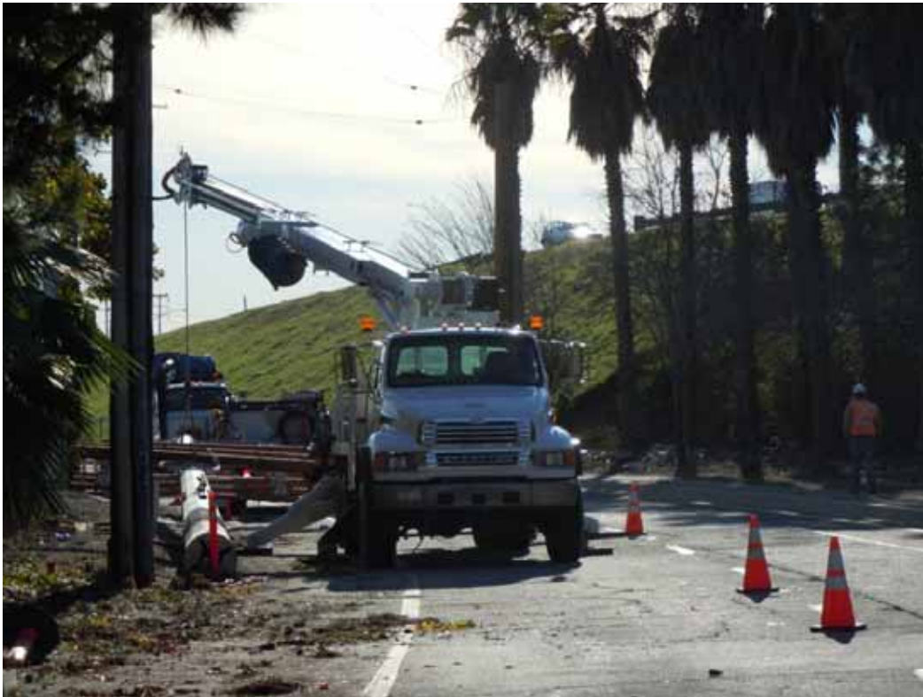
Figure 3: A Wilson crew prepares to install a LWSP along Rivergrade Road, Segment 7 66 kV.
