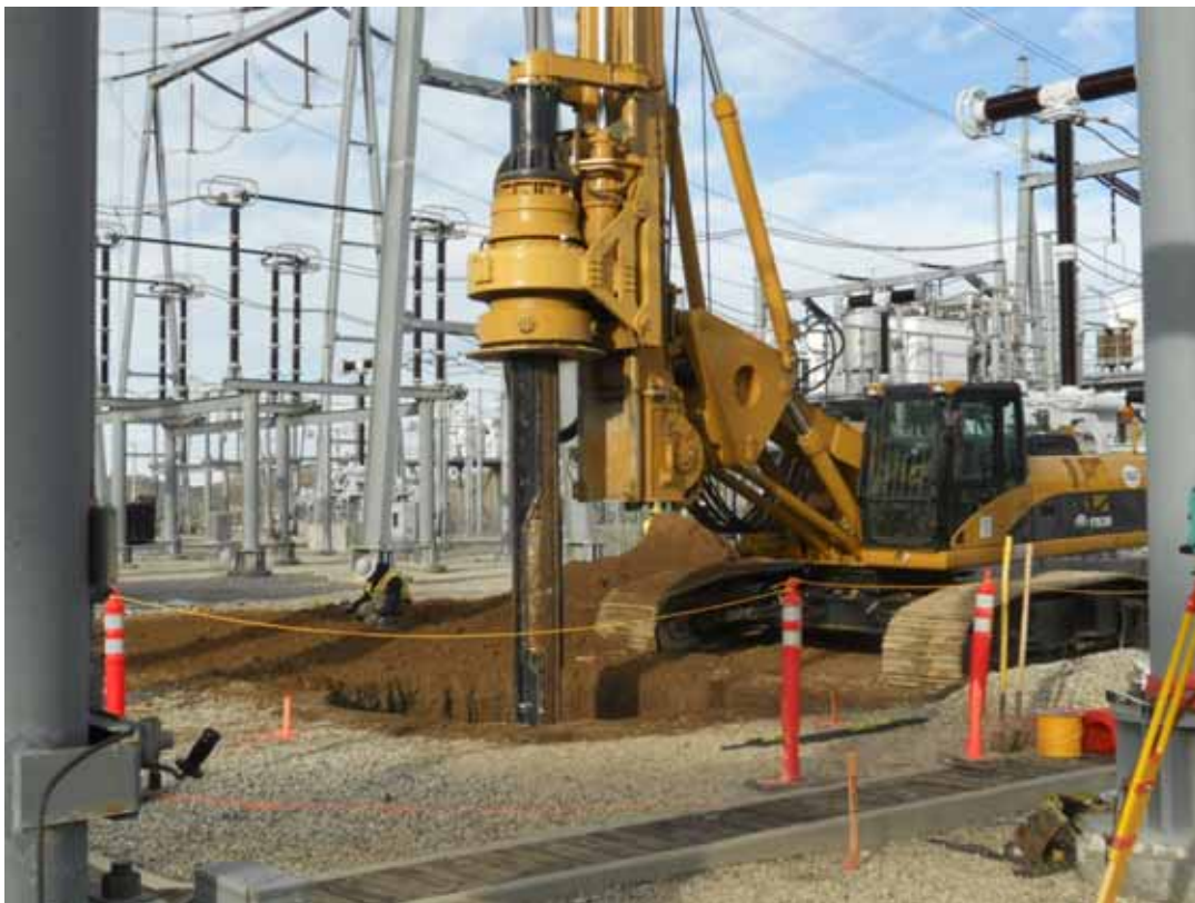
Figure 2: Woodward drilling Tower 71, (a TSP inside the Vincent Substation) with a Paleontological Monitor present, Segment 5.
