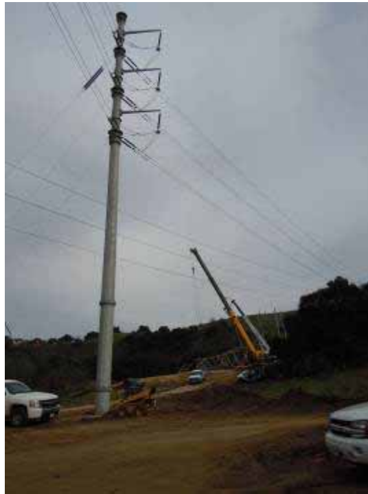
Figure 7: Crews work on erecting a tower at the M57-T3 shoofly, Segment 8 Phase 1, Tonner Canyon.
