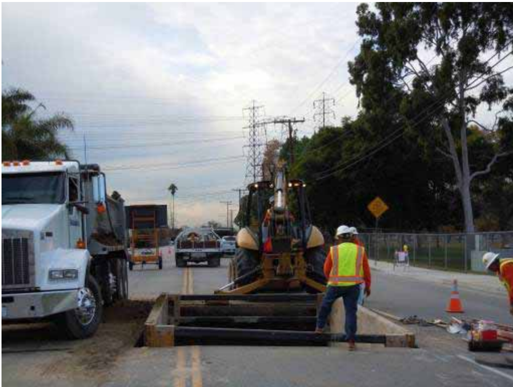
Figure 5: A Wilson crew sets a vault along Durfee Avenue, Segment 7, 66 kV underground portion.
