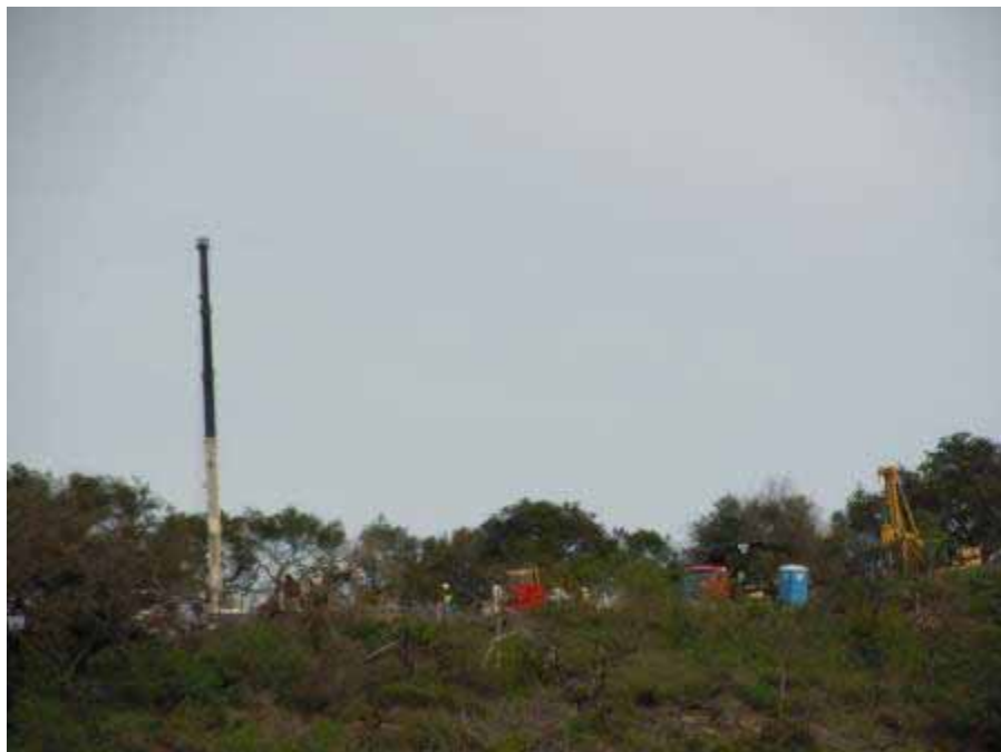
Figure 6: Crews work on the foundation for Tower M57-T4, Segment 8 Phase 1, Tonner Canyon.
