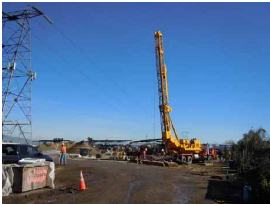
Figure 8: A Tri-State crew drills the foundation for Tower M1-T3, Segment 8, Phase 2, near Chino.
