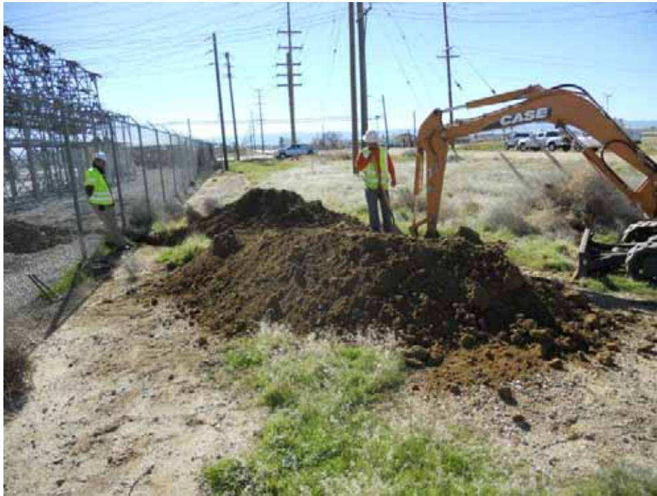
Figure 5: H&M crew trenching for underground FOC placement outside the Rosamond Substation, Segment 10 Telecom.
