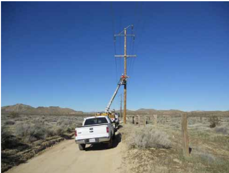
Figure 2: H&M crew installing cable arms on existing wood poles to support the telecom fiber optic cable (FOC) on 90 th Street, Segment 10 Telecom.
