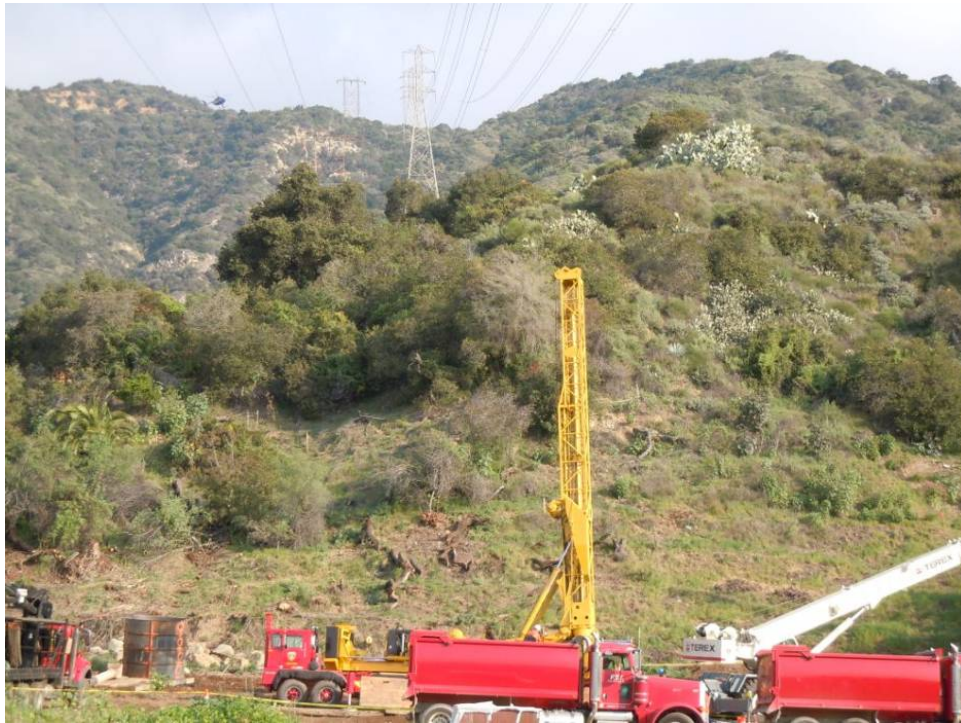
Figure 7: Crews work on the foundation for Tower M54-T3a in the foreground while a Wilson helicopter drops a lineman off at a tower in the background, Segment 7.
