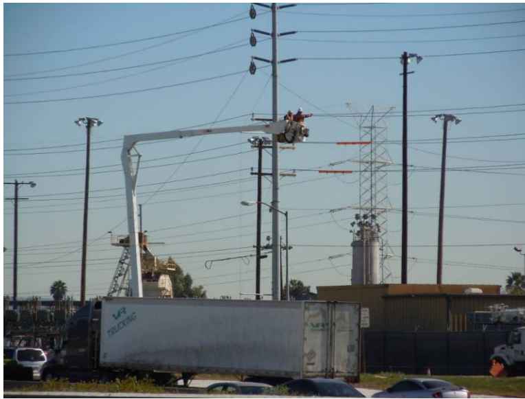
Figure 5: Crews transfer wire on the Rio Hondo–Amador-Jose-Mesa line in the City of Irwindale.
