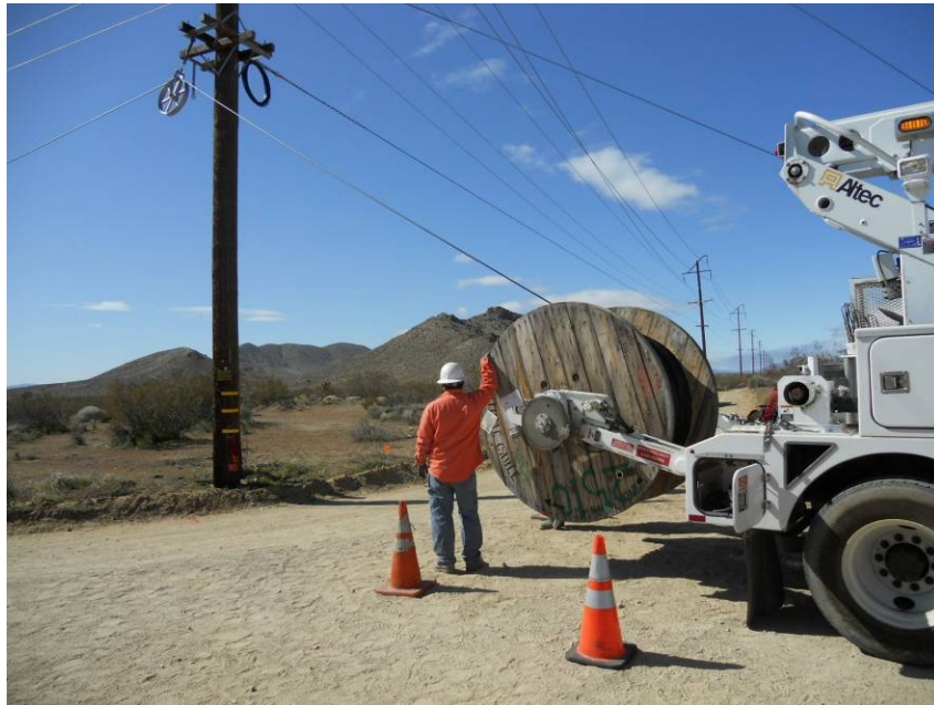
Figure 2: H&M crew pulling fiber optic cable (FOC) along 65 th Street, Segment 10 Telecom.
