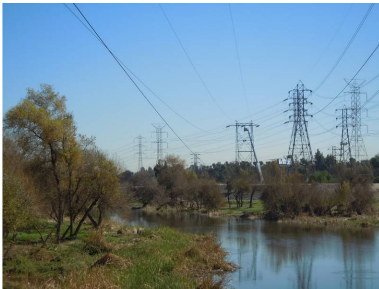
Figure 6: Crews remove conductor over the San Gabriel River in the City of El Monte, Segment 7.
