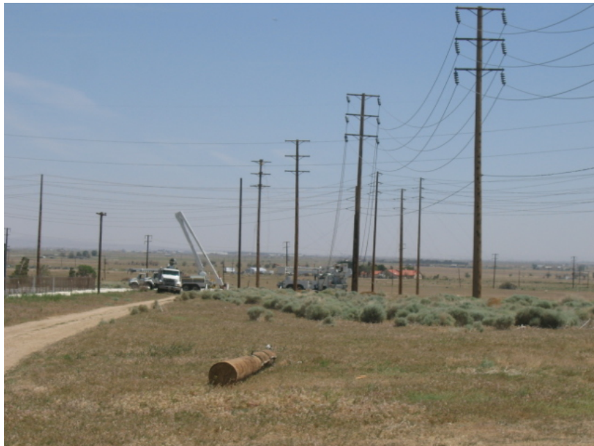
Figure 2: At the Antelope Substation, wood pole relocation took place in preparation for the substation expansion.
