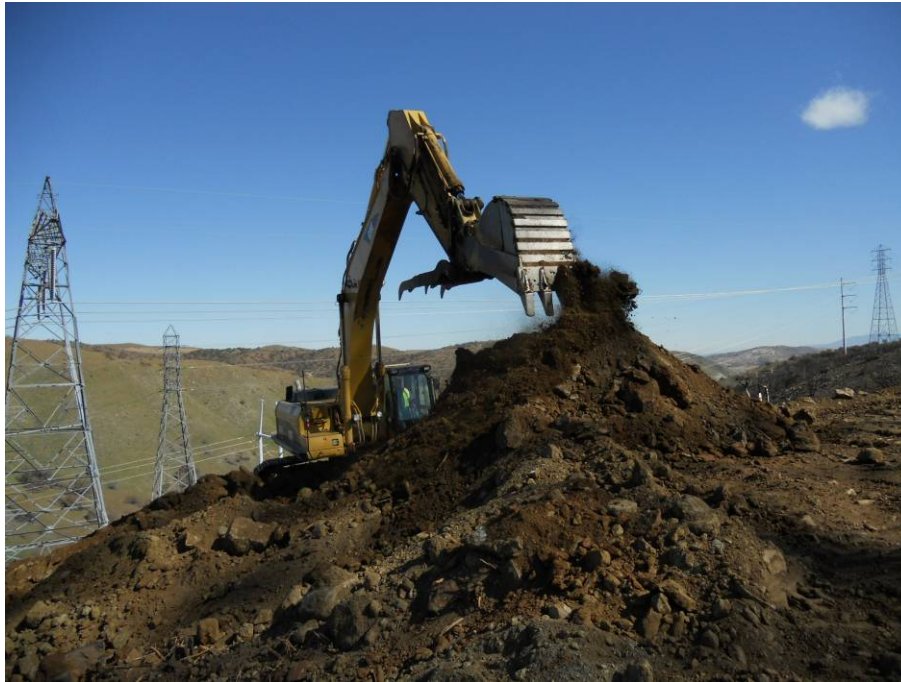
Figure 1: H&H grading disturbance site at Tower 30, Segment 5.
