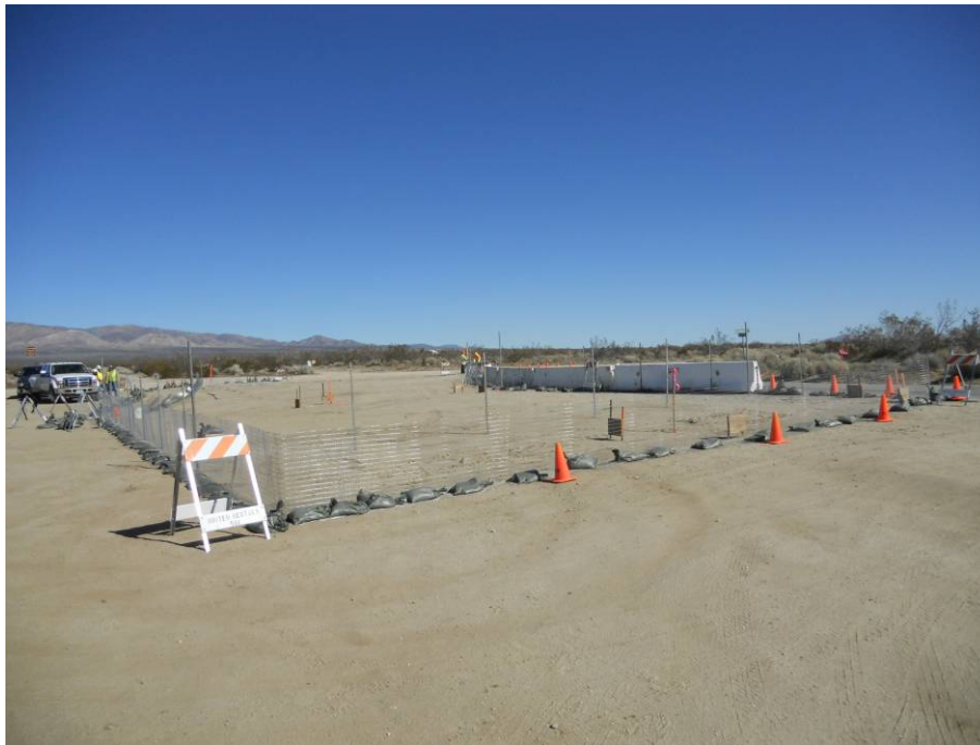
Figure 4: Temporary tortoise fencing in disturbed area along Rosamond Boulevard and 170 th Street at Whirlwind Substation, Segment 9.
