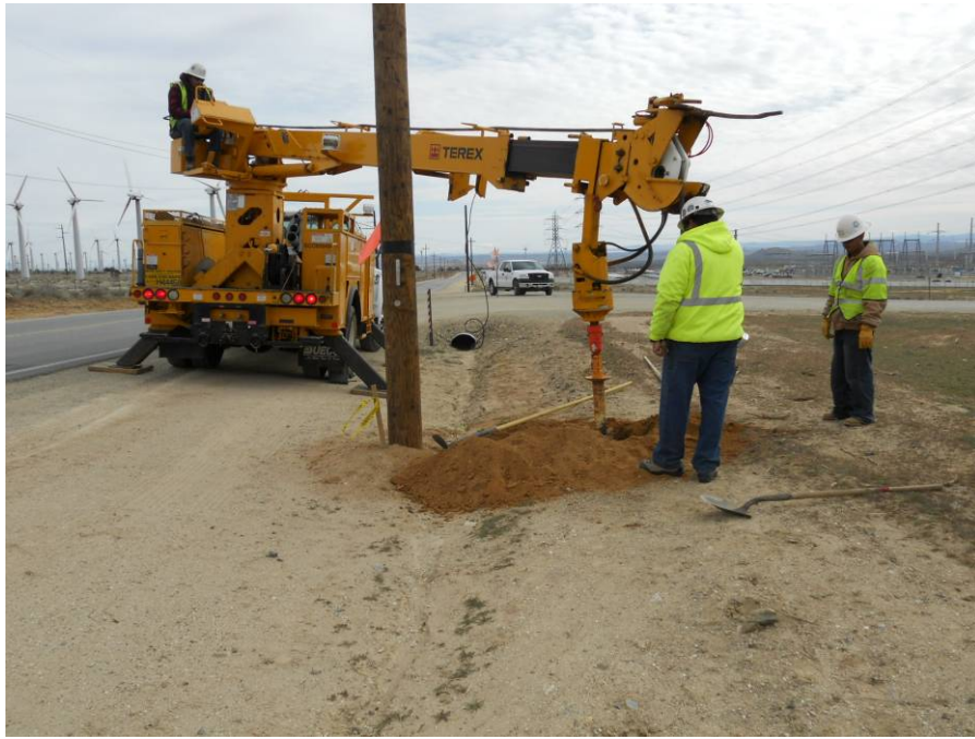
Figure 3: H&M crew relocating wood poles outside the Oak Creek Road drainage ditch, Segment 10 Telecom.
