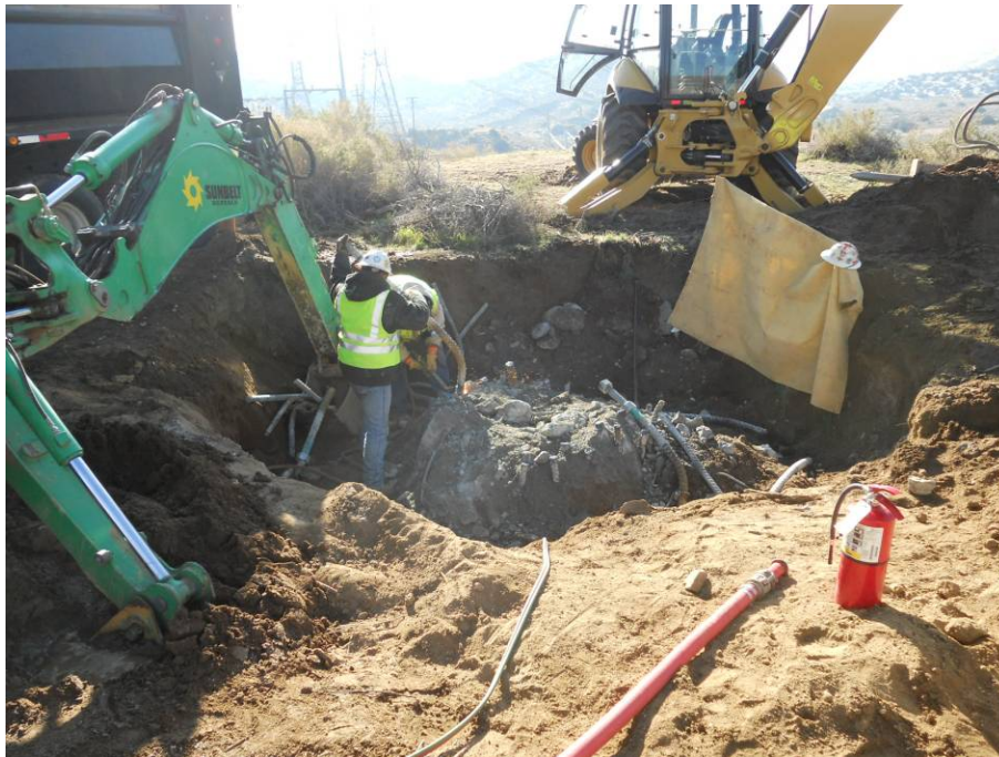
Figure 2: H&M crew removing old tower foundations near TSP 1 in the Vincent Expansion area, Segment 5.
