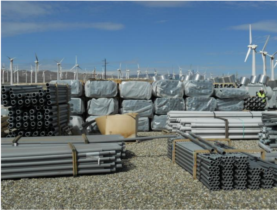
Figure 1: Plastic covering materials in Windhub Substation as bird deterrent, Segments 1-3.
