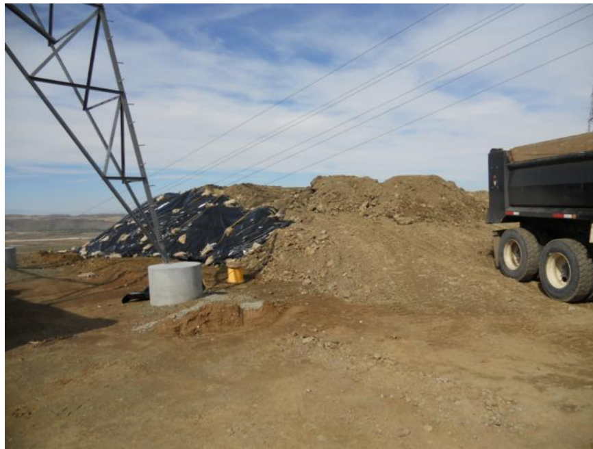
Figure 3: Soil from new access road grading at Tower 42 being stockpiled at Tower 41, Segment 5.
