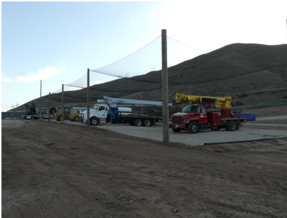
Figure 4: Netted parking area to deter nesting birds in Vincent South Material Yard, Segments 6 & 11.
