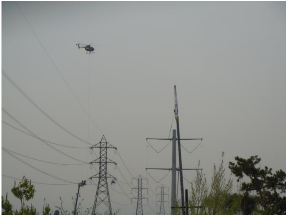
Figure 6: Crews erecting a double circuit TSP in the City of Duarte, Segment 7.
