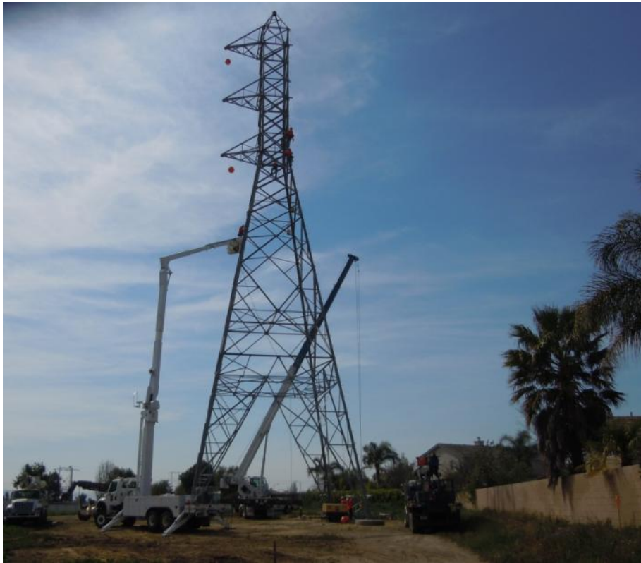
Figure 7: Crews erect a double circuit lattice steel tower (LST) in the City of Chino, Segment 8, Phase 2.
