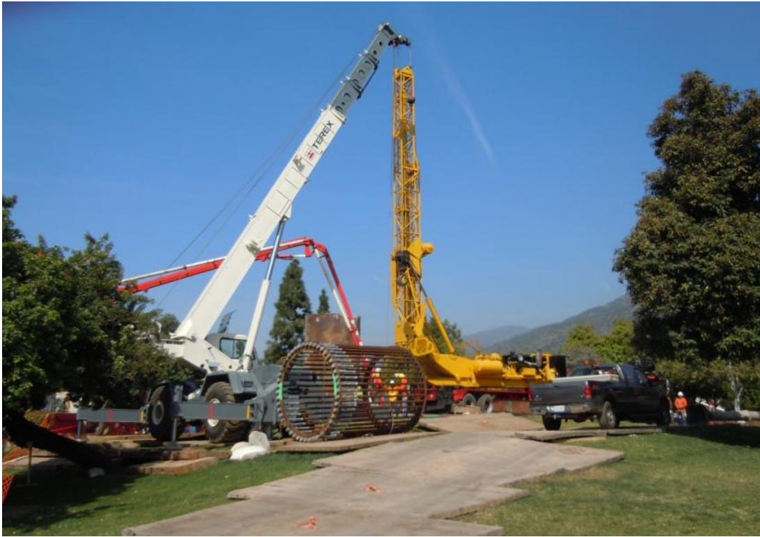
Figure 5: Crews pouring concrete at a TSP foundation within Hacienda Park in the City of Duarte, Segment 7.
