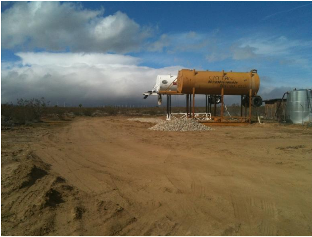
Figure 3: Cattracs (Whirlwind grading contractor) water tower placed on private property adjacent to Backus Road.
