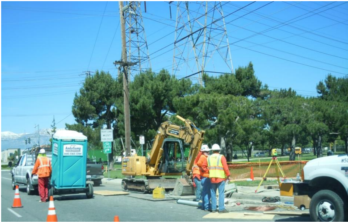
Figure 5: Crews work on a riser foundation, Segment 8 66 kV in the City of Chino.
