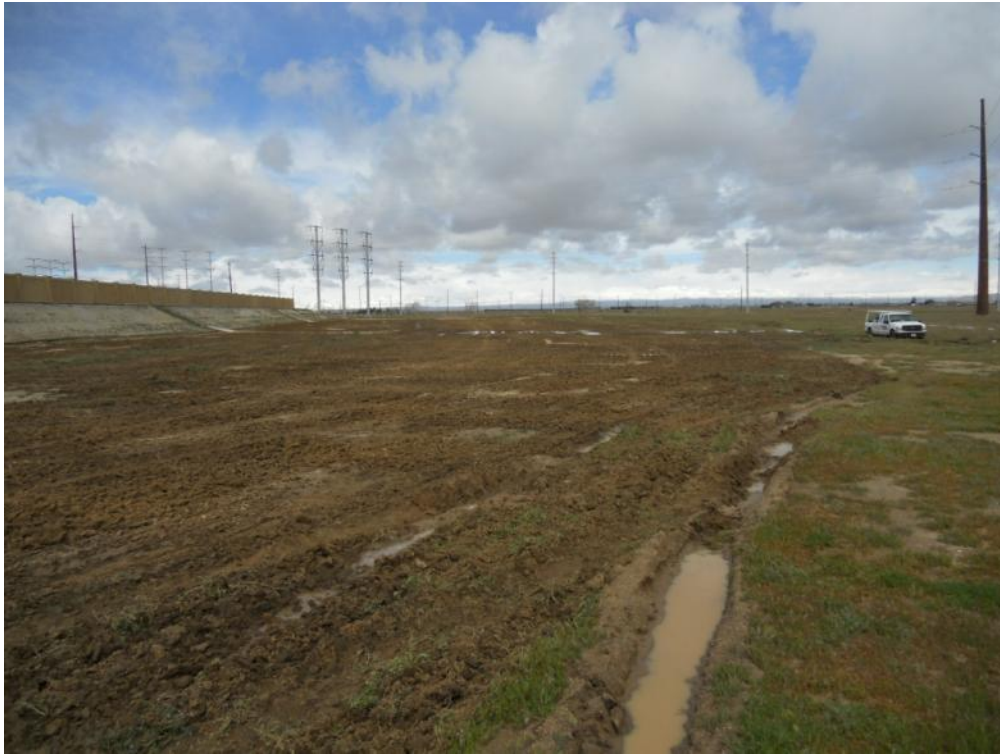
Figure 1: View of the east side of the Antelope Substation expansion that was recently prepped for seeding.
