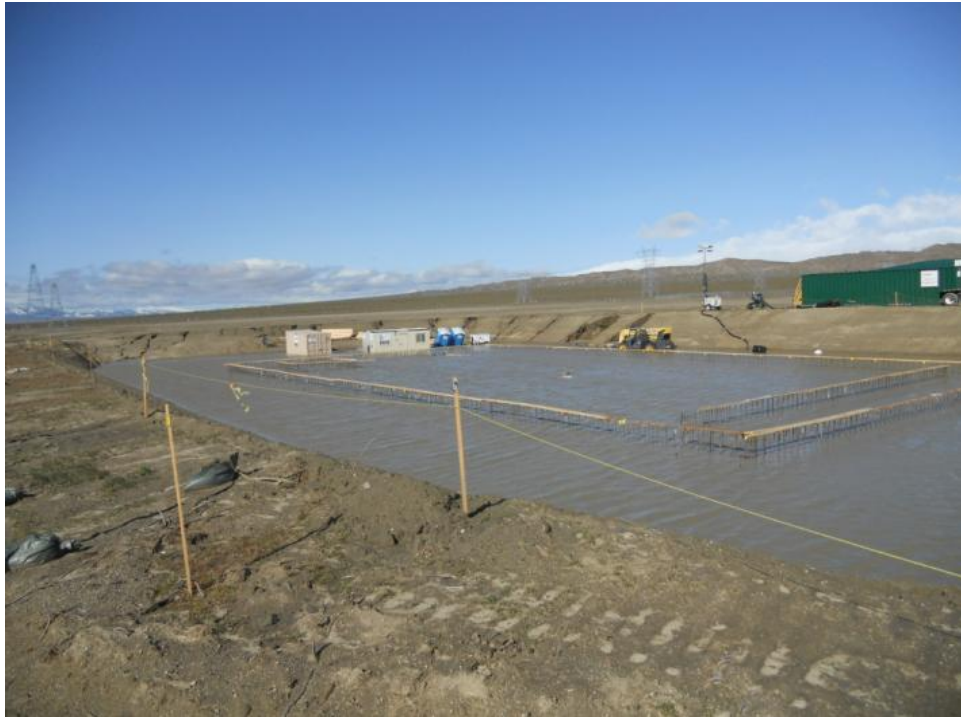
Figure 4: MEER excavation with 3-feet of stormwater in Whirlwind Substation, Segment 9.
