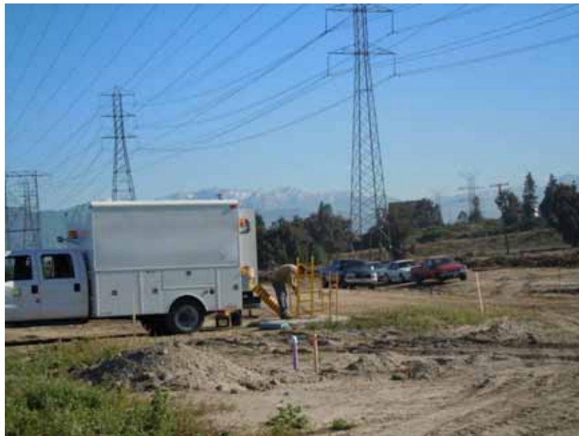
Figure 6: SCE crews pull conduit within the Duck Farm, Segment 7 66 kV, City of South El Monte.
