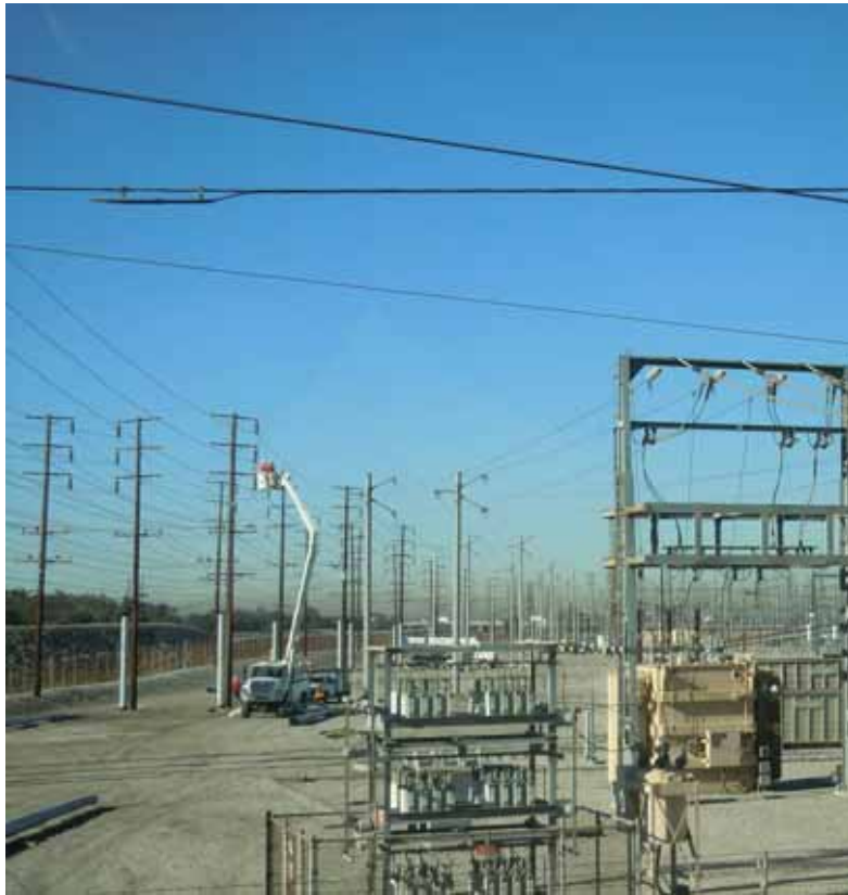
Figure 5: Crews work reframe conductor within the Rio Hondo substation, Segment 7 66 kV in the City of Irwindale.
