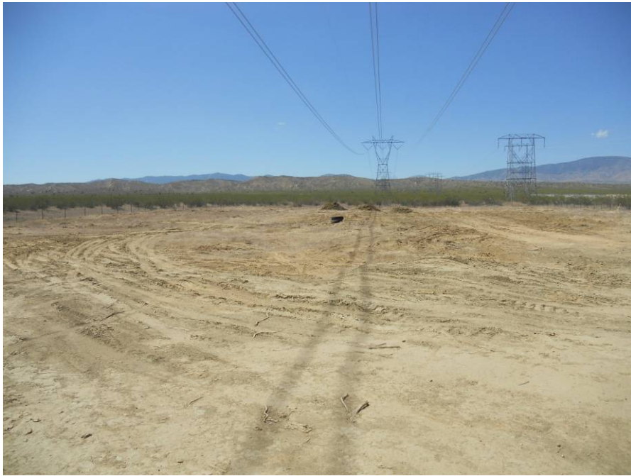
Figure 3: View north of the cleared pull site at Tower M73-T3A outside the Whirlwind Substation, Segment 4.
