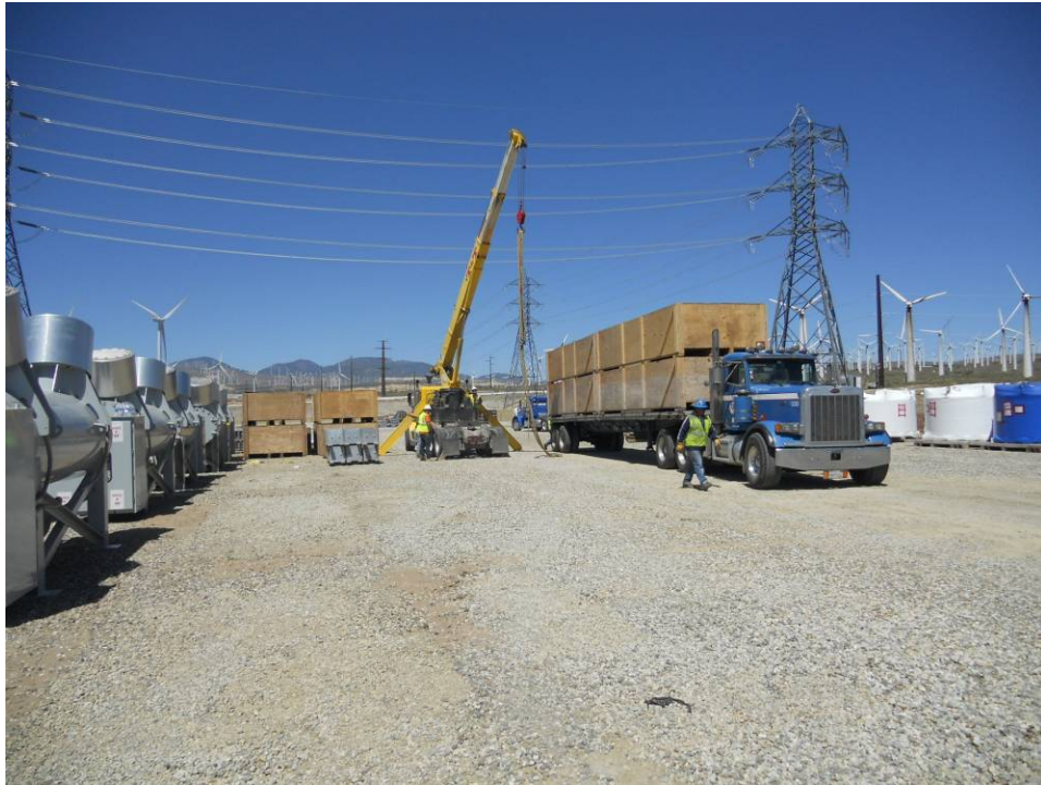
Figure 1: Materials being loaded in Windhub Substation that will be transported to Whirlwind Substation, Segments 1-3.
