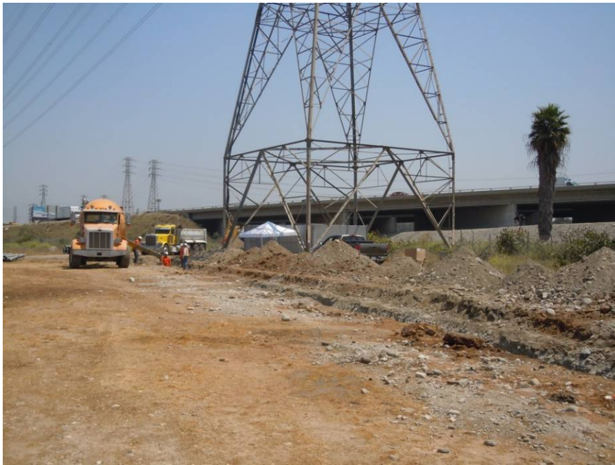
Figure 5: Crews pour slurry into the trenchline for the Rio Hondo–Anita No. 2 underground adjacent to the I-605 freeway, Segment 7 66 kV.
