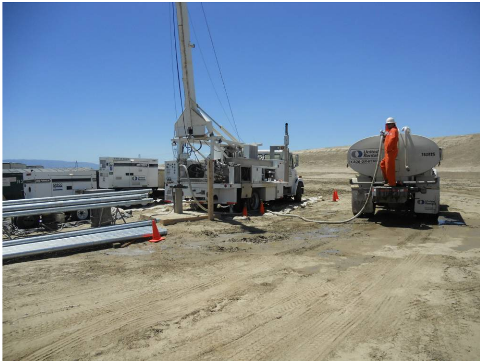
Figure 3: The onsite well inside the Whirlwind Substation, Segment 9.
