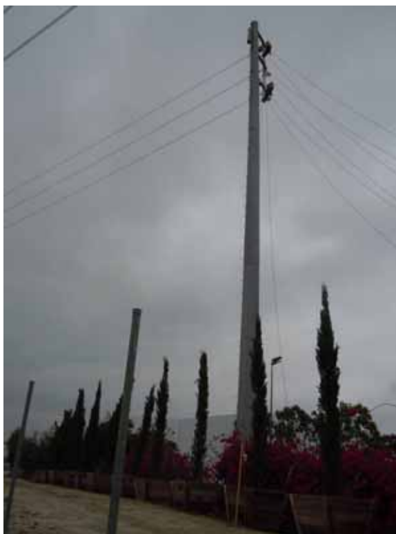
Figure 5: SCE crews string wire on the overhead Rio Hondo–Amador-Jose-Mesa line, Segment 7, 66 kV.
