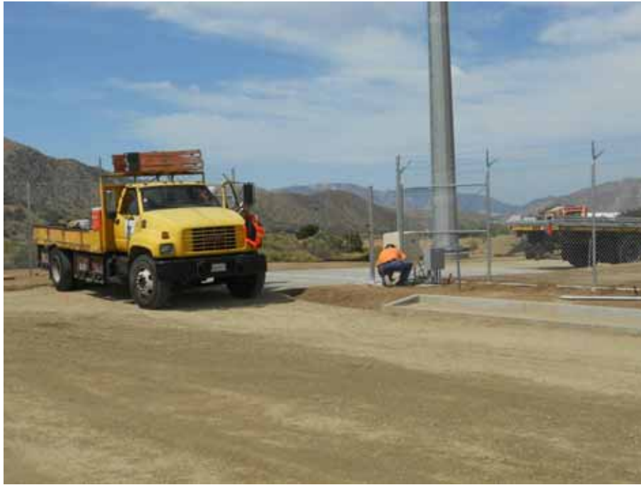
Figure 1: Gate installation at the perimeter fence around the Vincent Substation Expansion, Segment 9.
