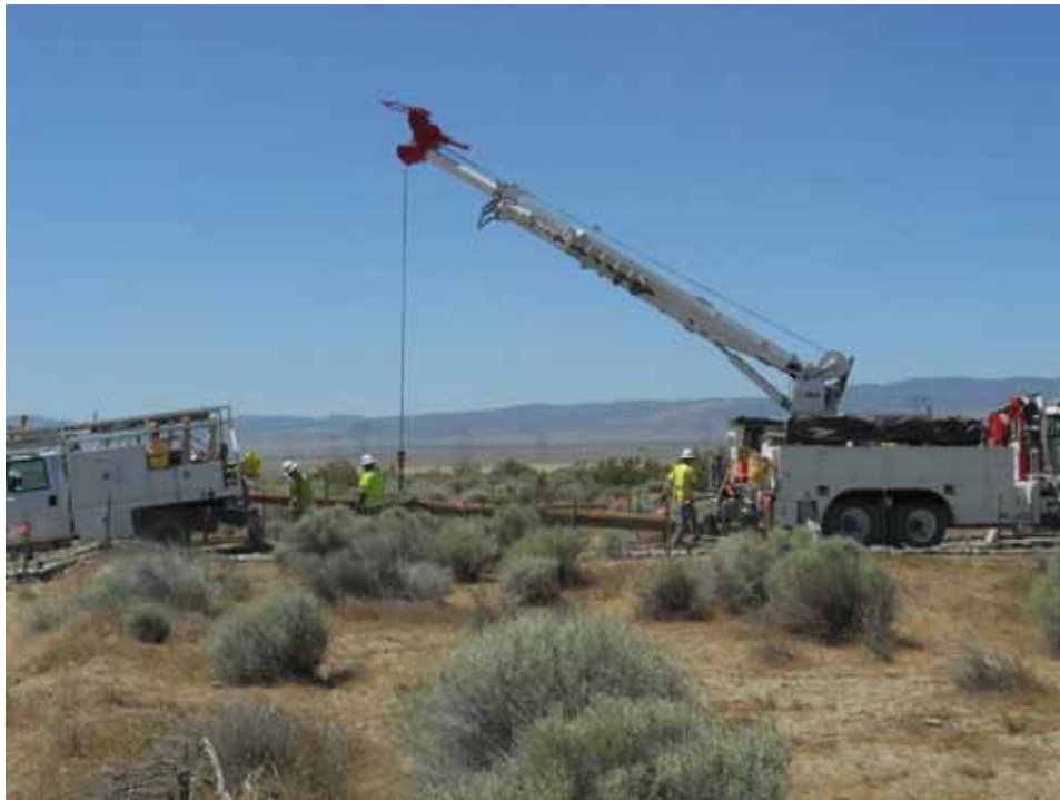
Figure 3: SCE crew preparing to set a wood pole outside Whirlwind Substation on the west side of 170 th Street, Segment 10 Telecom.
