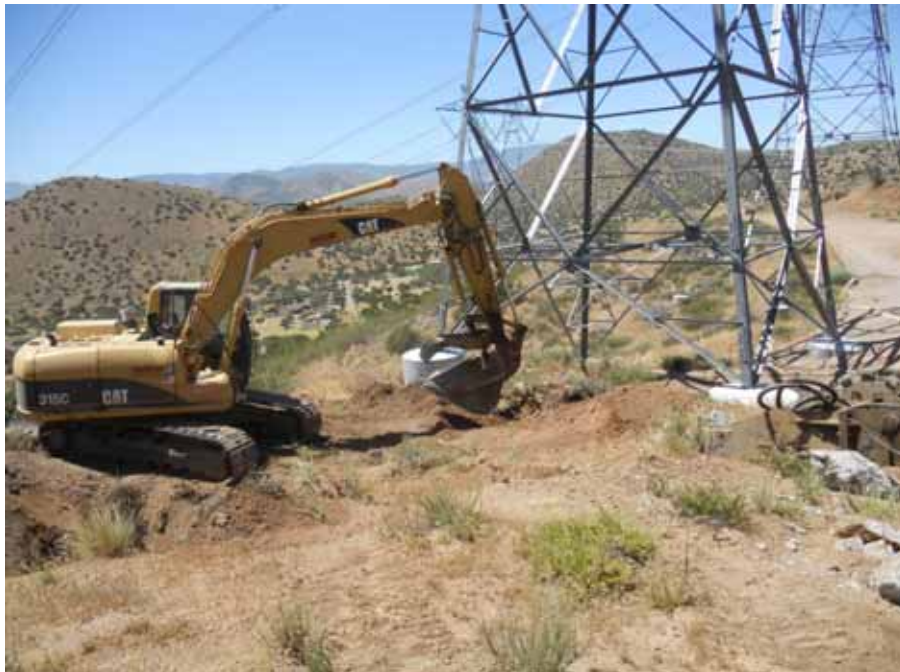
Figure 2: H&H Grading removing old 220 kV tower foundations near new 500 kV Tower 60, Segment 5.
