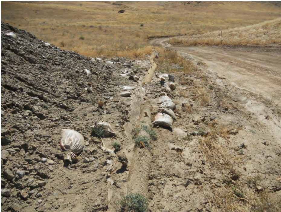
Figure 4: BMP's in disrepair around soil stockpile near Tower 41, Segment 5.
