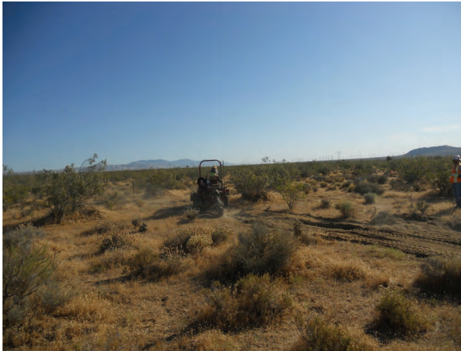
Figure 3: Moore Fence crew using a ditch witch to install tortoise fence at Tower 42, Segment 10.
