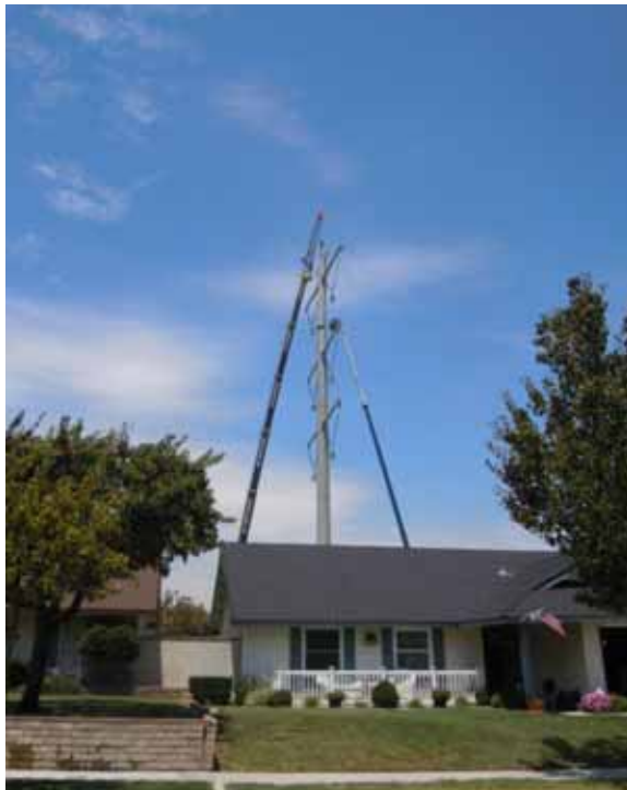
Figure 7: A Wilson crew sets the top segment of a TSP in Chino Hills, Segment 8 Phase 1.
