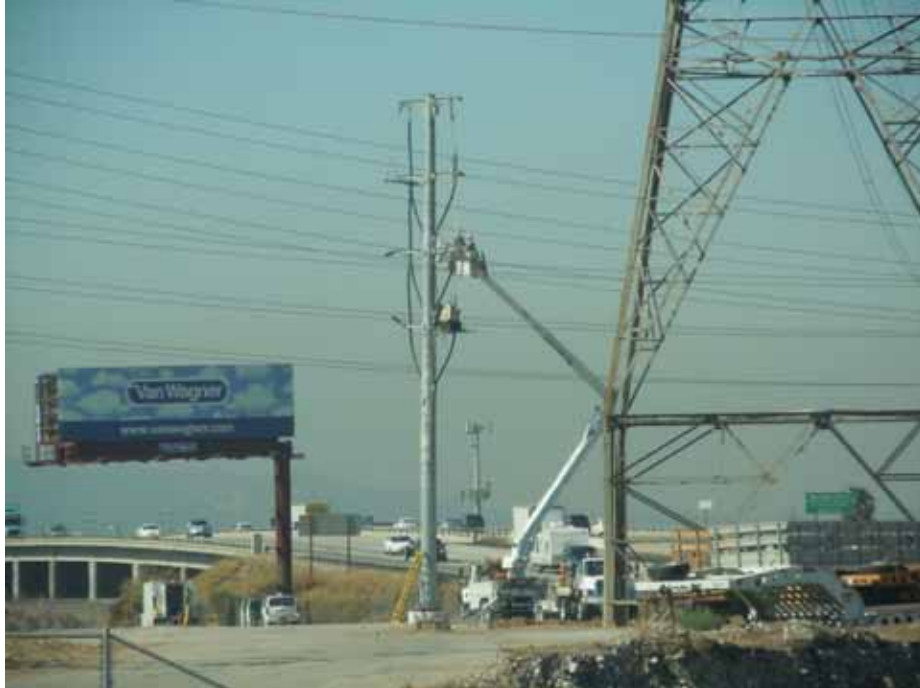
Figure 6: A 66 kV crew works on a riser pole on the Rio Hondo–Amador line, Segment 7.
