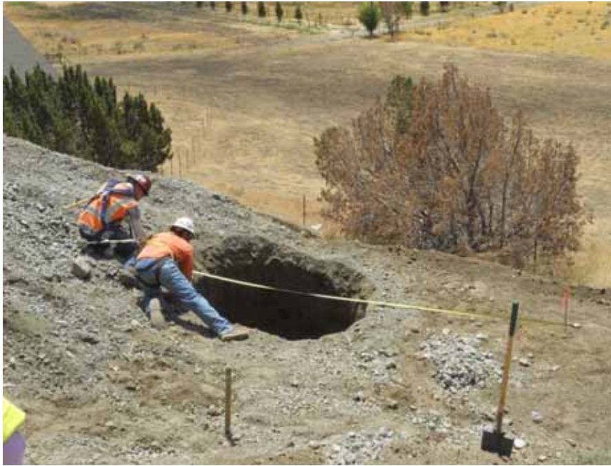
Figure 1: Woodward driller and Burns & McDonnell Inspector measuring foundation hole at Tower 28A, Segment 5.
