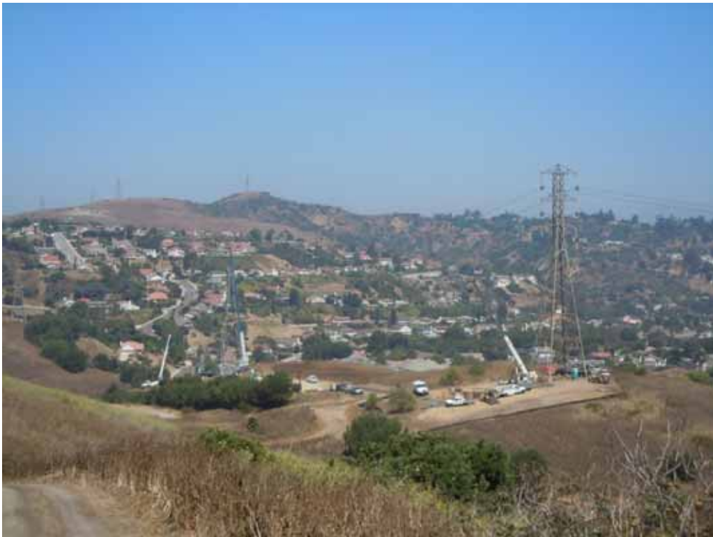
Figure 9: A DCX crew drills a 500 kV foundation (foreground) as a Wilson crew assembles a 220 kV interset tower (background), Segment 8 Phase 4.
