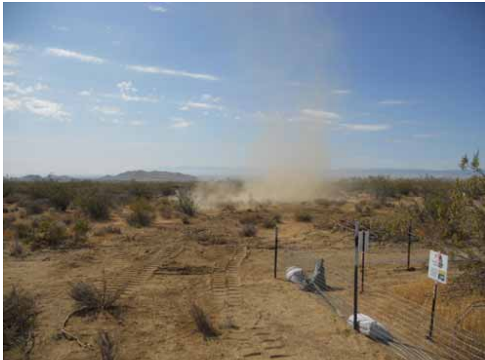
Figure 4: Fugitive dust from chipping activity at Tower 50 (no prior watering of site), Segment 10.
