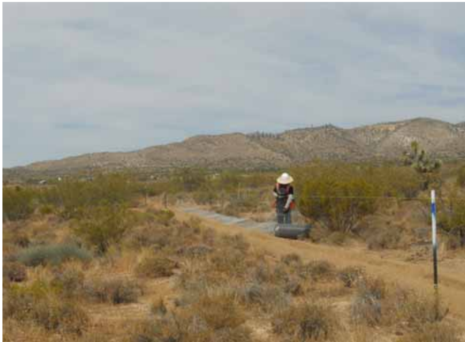
Figure 2: Moore Fence crew member rolling out the tortoise fence along the wire setup site at Tower 29, Segment 10.
