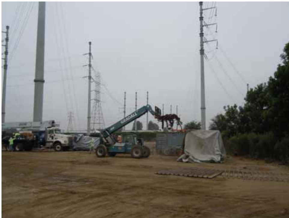
Figure 8: Crews dispose of construction waste at the I-605 Shoofly disturbance area, Segment 8 Phase 4
