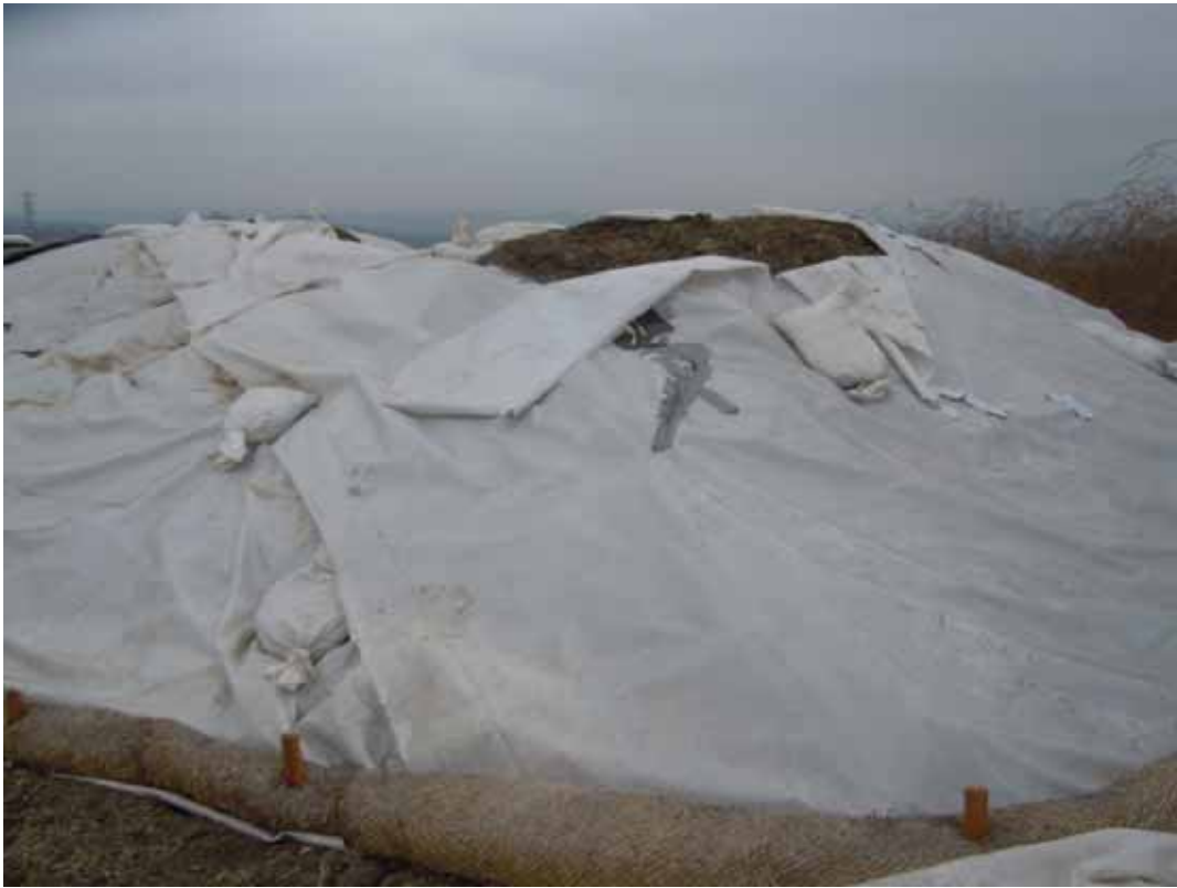
Figure 11: Torn plastic atop a soil pile, Segment 8 Phase 4.
